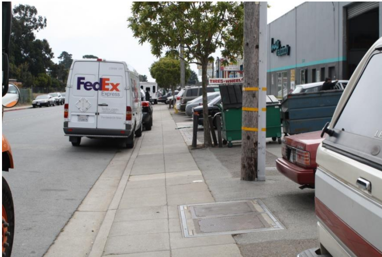
Photo 26, 27 & 28 Old Mission Road west, Driveways/sidewalk does not meet ADA Standards for path of travel
