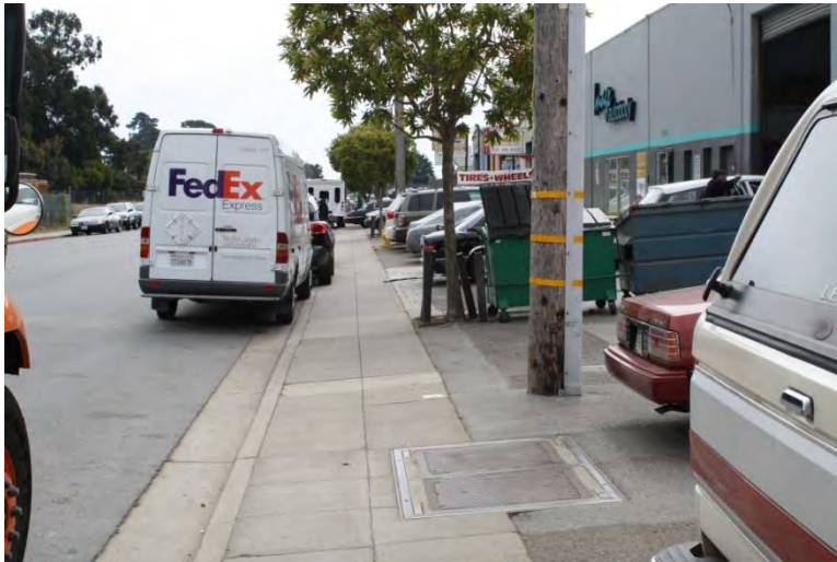
Photo 26, 27 & 28 Old Mission Road west, Driveways/sidewalk does not meet ADA Standards for path of travel
