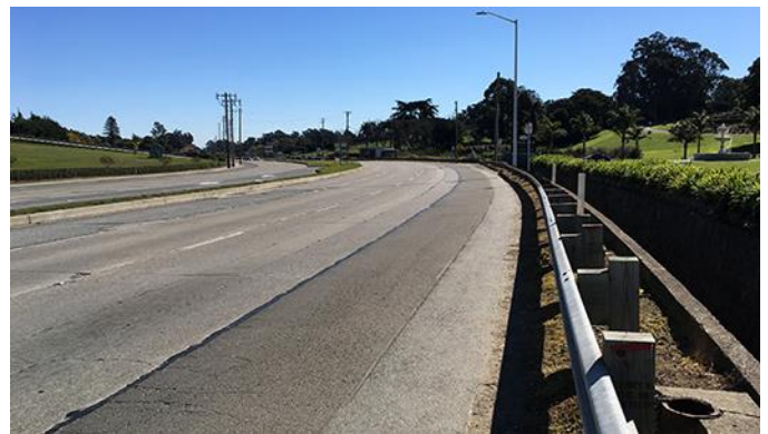
Missing sidewalk and Bike lane northbound, westside of ECR, in front of Woodlawn/Creek Orthodox Memorial Park
