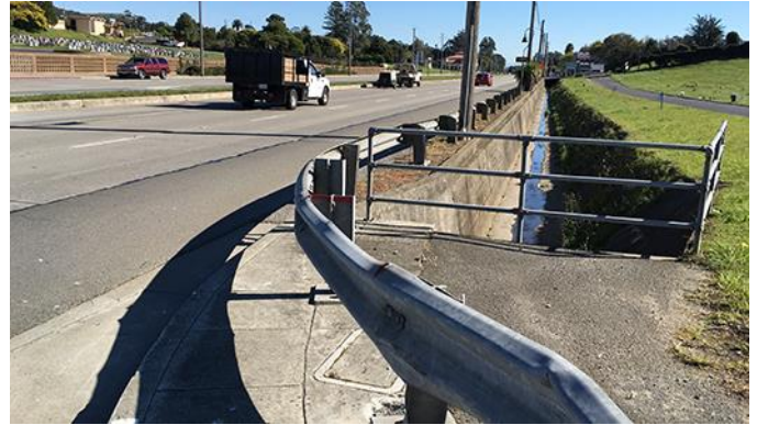
Missing sidewalk and bike path northbound, on westside of ECR, next to the open cement channel
