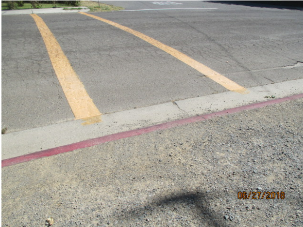
Missing Pedestrian Ramp at the Westerly Crosswalk of Prune Street Intersection
