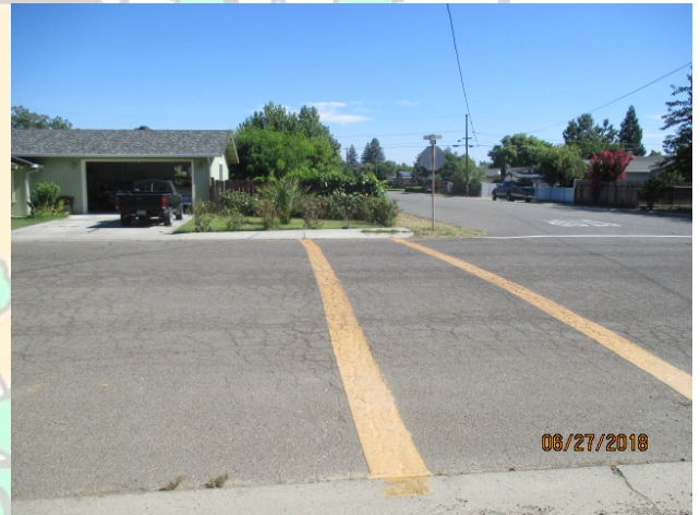
Westerly Crosswalk and Inadquate Pedestrian Ramp at Prune Street Intersection
