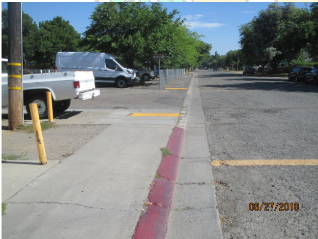
Missing Pedestrian Ramp at Hickory Street Intersection
