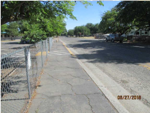
Missing Sidewalk looking North on Fig Street
