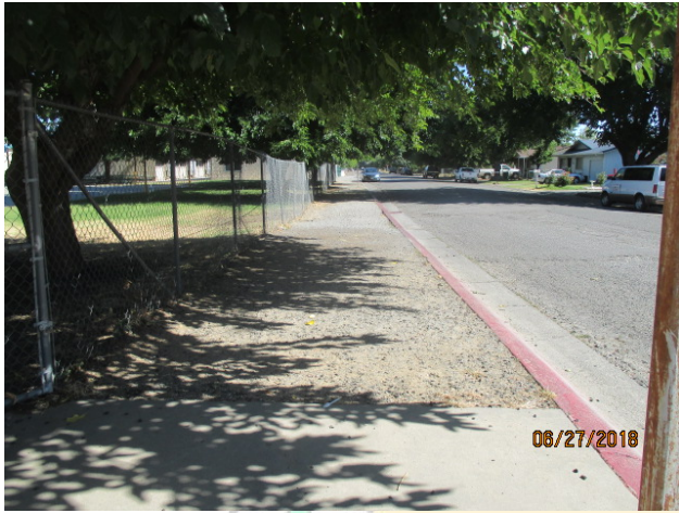
Missing Sidewalk North of Fig Lane Intersection
