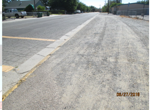
Missing Sidewalk and Pedestrian Ramp on the Easterly Crosswalk at Prune Street Intersection
