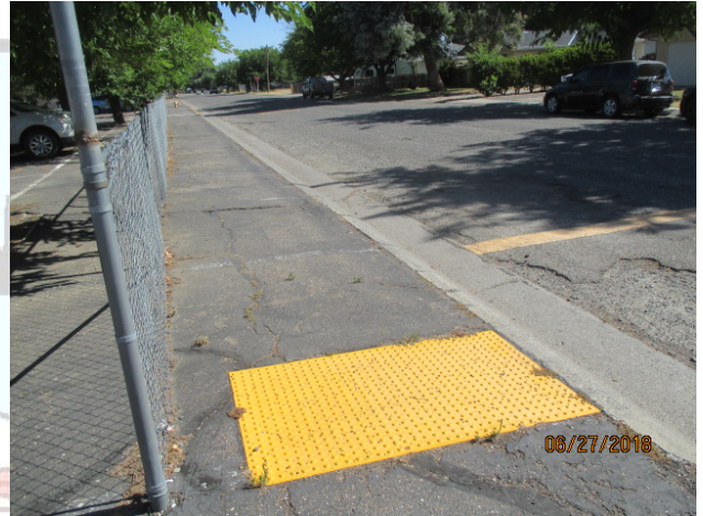
Missing Pedestrian Ramp and Sidewalk North of Hickory Street Intersection
