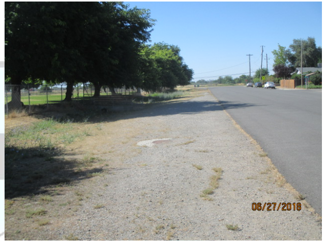
Missing Sidewalk on East Side of Pear Street
