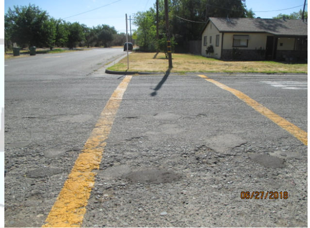
Existing Crosswalk and Missing Pedestrian Ramp looking East at Almond Street Intersection
