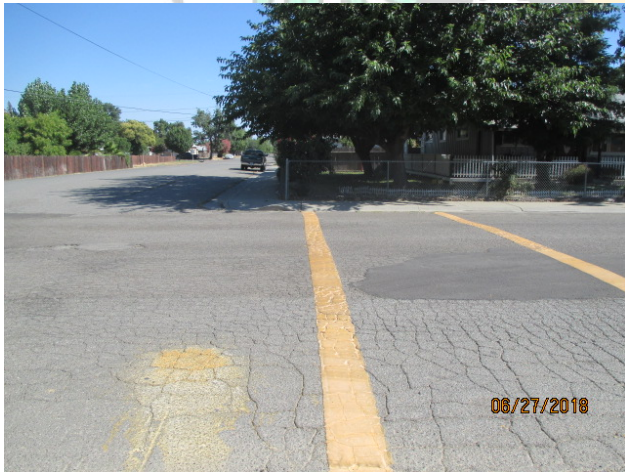
Easterly Crosswalk and Inadquate Pedestrian Ramp at Prune Street Intersection
