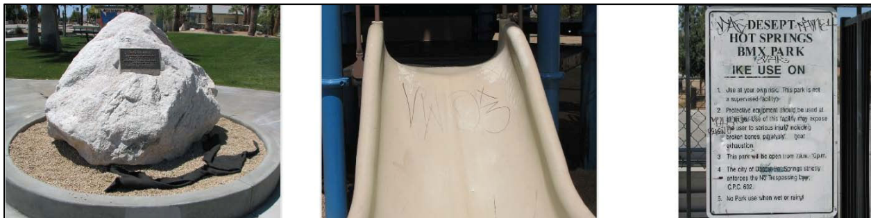
A variety of maintenance issues were observed during site visit of park sites.
