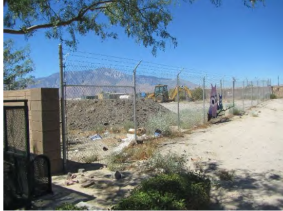
Photograph 6 – Photograph showing the construction staging area located on the northeastern portion of the subject property.
