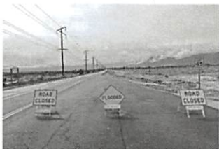
Flooding caused by heavy rain on Friday night and Saturday morning closed Little Manzanita Road in Desert Hot Springs.
