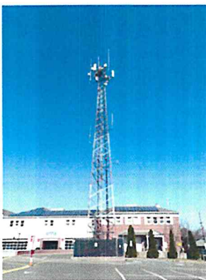
Non-concealed Tower: radio heads and antenna are visible. *Picture taken at 1 Cedar Street Emergency Communications Center.
