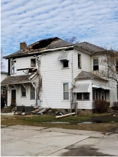
A fire at 605 West Fayette Ave in February caused extensive damage. Firefighters rescued family pets. No injuries were reported.
