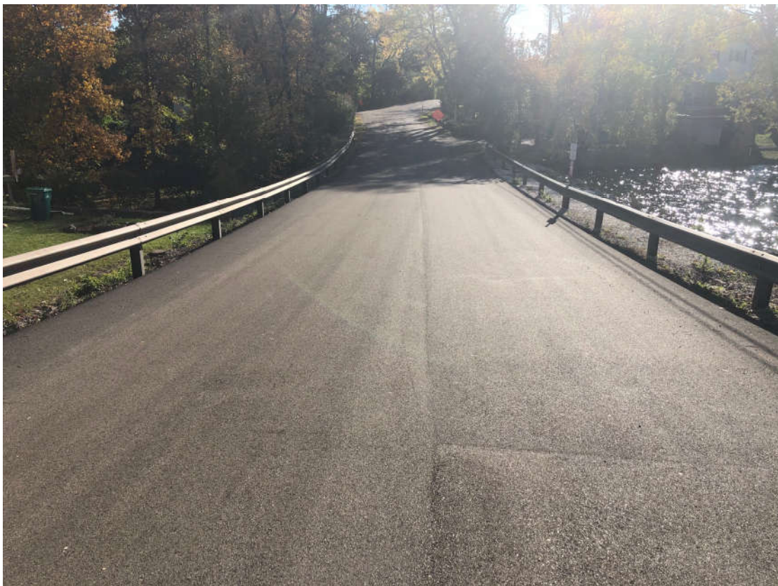
Lakeside Drive- 11/1/2021 (Forest Lake on right side of road, outlet pipe on left side)
