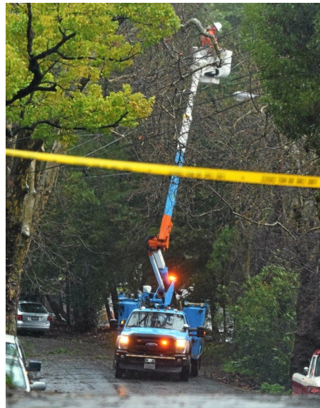
Figure 183: Wind Damage on Spruce Road – 2017 Storm
