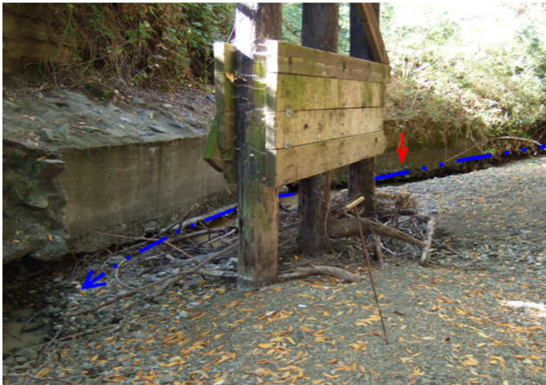
View upstream to right bank showing area of focused bed scour along the toe of the right bank and near Pier 4. The concrete toe wall bank protection structure at the outside bend channel position is undercut by as much as 4 horizontal feet
