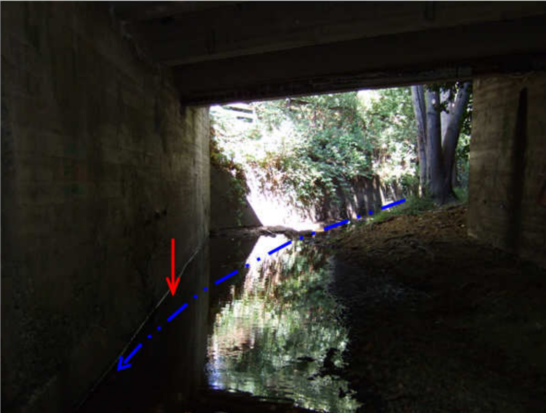
View upstream through the bridge showing bedrock outcrop at the left abutment wall and scour
