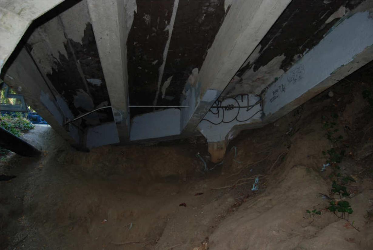
Minor, inconsequential erosion cause by foot traffic at Abutment 5
