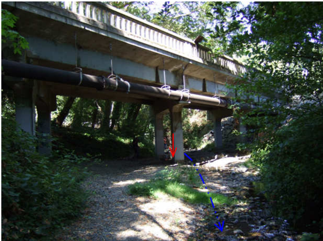
View upstream from the channel centerline to the area of scour focused along the center bridge pier
