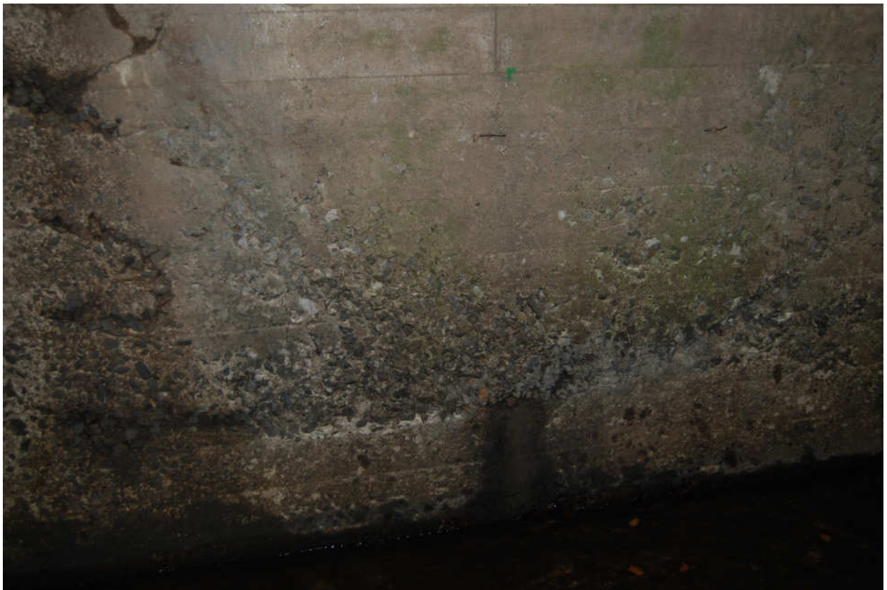
In spite of the poor concrete quality the long abutment will sustain the span above for some time to come.
