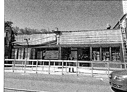
IMAGE: CURRENT (MANSARD REMOVED FOR SAFETY REASONS)
