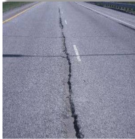
Transverse or Longitudinal Cracking
