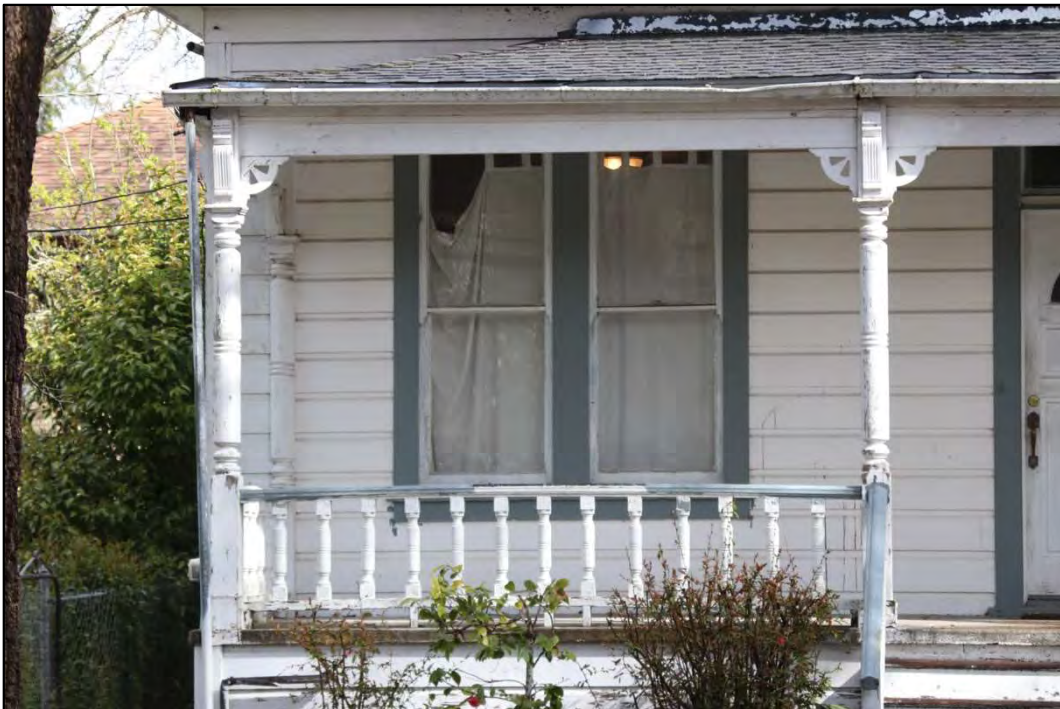
Figure 4: South elevation, pair of windows at SW corner, balustrade and porch posts
