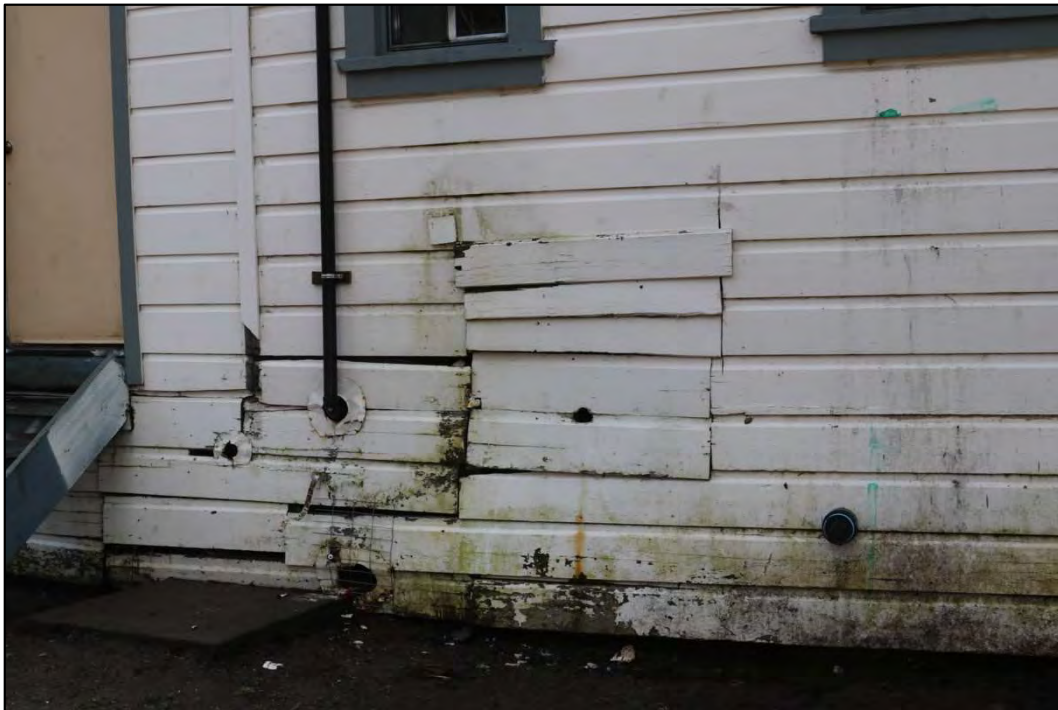
Figure 20: North elevation, patch
