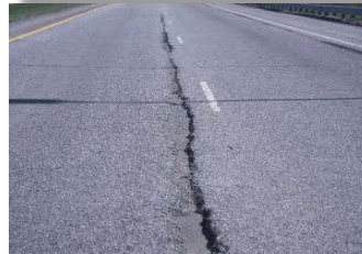
Transverse or Longitudinal Cracking
