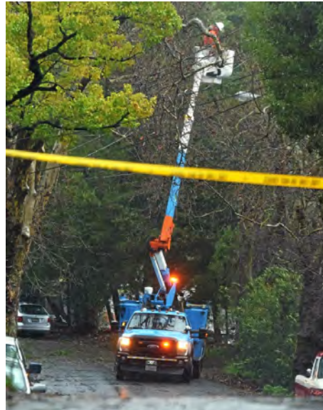
Figure 39: Wind Damage on Spruce Road – 2017 Storm
