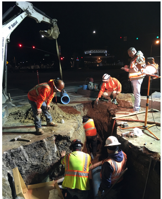
▲ Maintaining utility systems 24-7 [cover photo]
