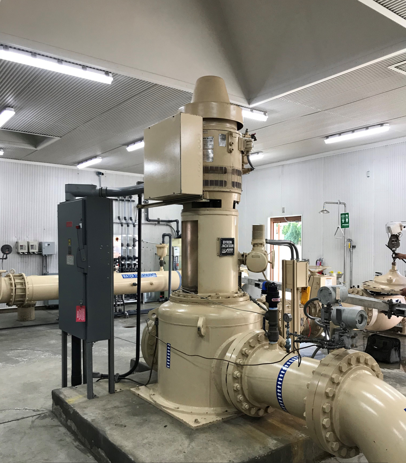
Hydropower: The City's Public Works Agency purchases millions of kilowatt-hours every year to operate well pumps and booster pumps to deliver clean water. The City continuously evaluates and implements onsite renewable energy systems (shown here is a hydropower project) to offset some of this electric load, lowering electric bills and reducing the associated greenhouse gas emissions.
