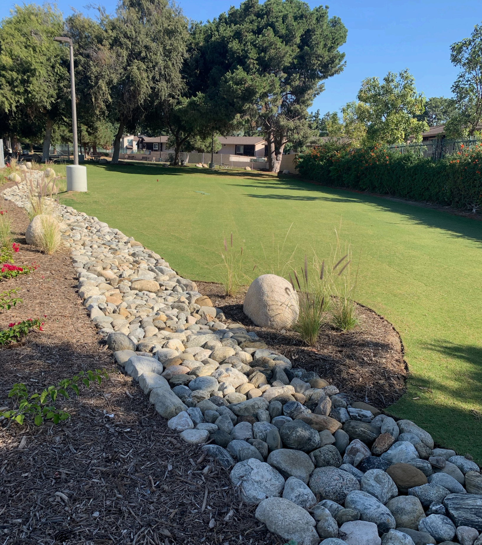
Mabury Park Stormwater Project. Completed in 2019, the project included the construction of a 7,000-square-foot bioretention basin designed to capture and infiltrate approximately 27,000 cubic feet of stormwater during a significant storm. The bioretention basin will capture stormwater runoff and use natural filtering through the soil to remove pollutants before it is released into the City's storm drain system. This project was the first regional stormwater infiltration best management practice (aka BMP) in the City of Santa Ana.
