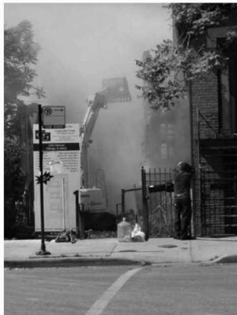
Photo 3. No dust suppression used at a demolition site in Chicago. Source: University of Illinois at Chicago
