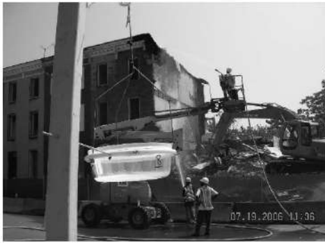
Photo 5. Extensive dust suppression used at a housing demolition site in Baltimore, with simultaneous water application to roof and to debris pile below. Lead dust fall sampler shown in foreground. Source: East Baltimore Development Initiative
