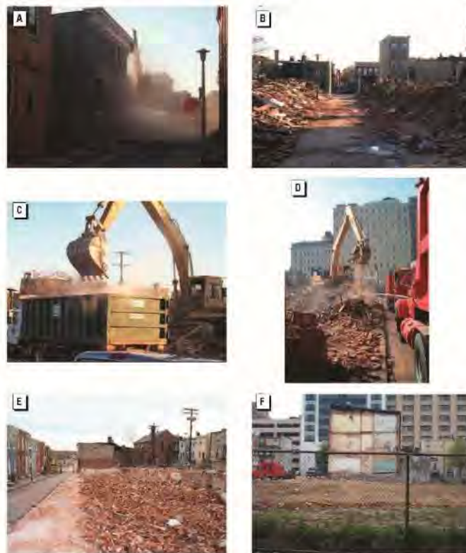
Figure 3. Demolition in progress. Site 1: (A) during demolition, (B) after demolition and before debris removal, and (C) debris removal. Site 2: (D) debris removal, (E) after debris removal, and (F) vacant lot.
