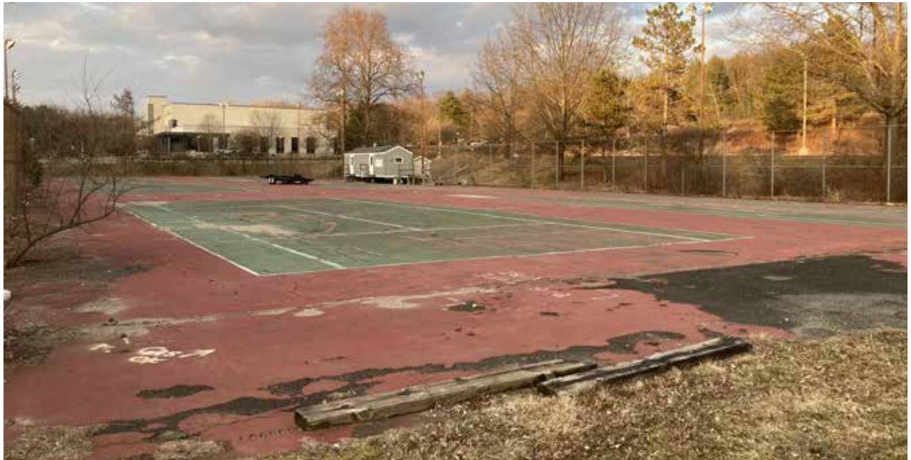
HCC tennis courts in disrepair.
