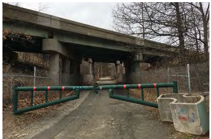
The dark walkway under I-91 to Anniversary Hill Park and Scott Tower (above, photo courtesy of Mark Roessler and the Valley Advocate) isolates the area from the popular and well-used Community Field Park (below, photo by Tamsin Flanders).
