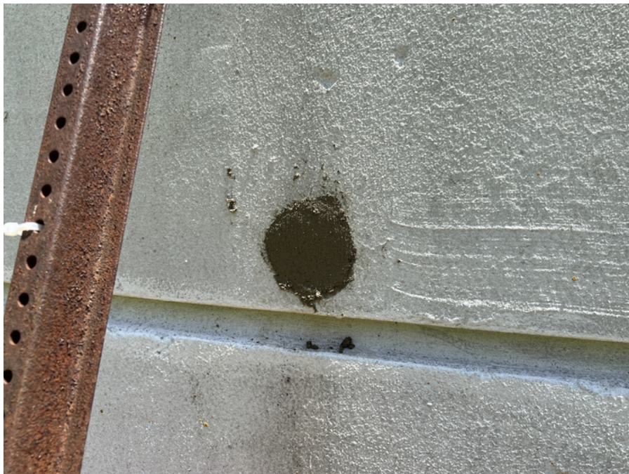
(P5) W-1 patch from outside
