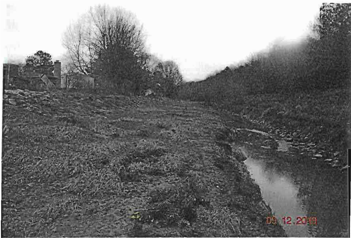
Looking up stream. Note blockage in creek and rip rap has fallen into water.
