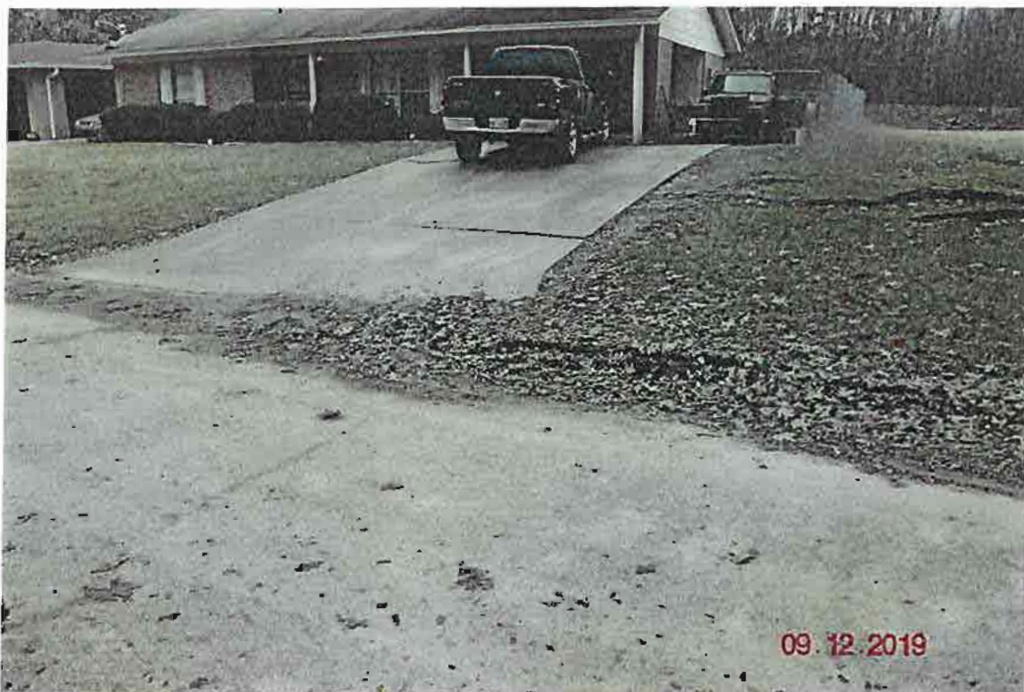
Drainage ditches downhill blocked. Clean out of concrete gutters needed.
