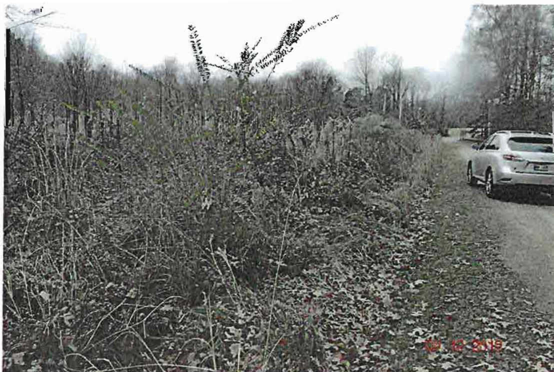
Blocked drainage ditches.
