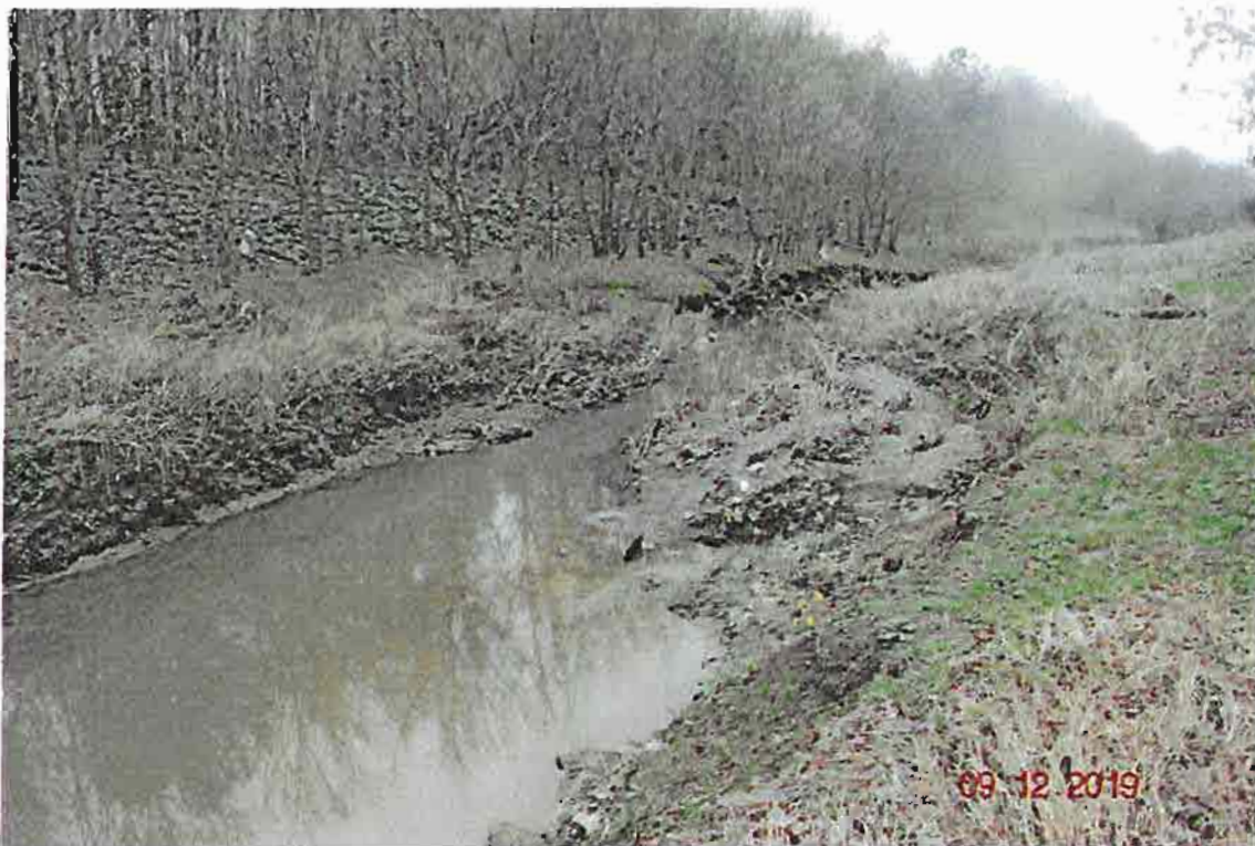
Looking down stream. Note blockage in creek. Lower rip rap now completely in creek.
