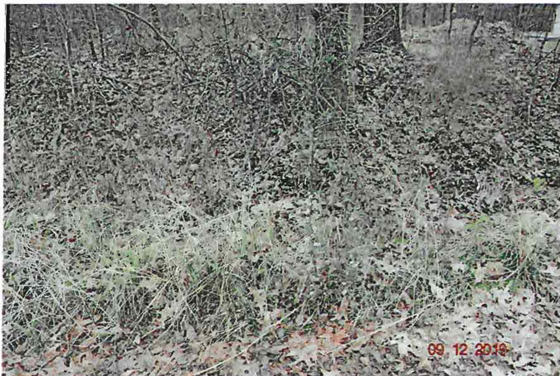
Blocked drainage ditches.
