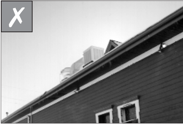
Minimize the visual impacts of mechanical equipment, as seen from the street.
