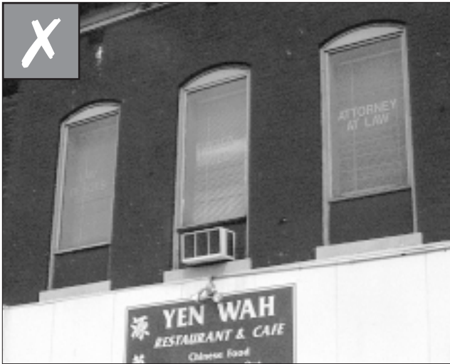
Installing window air-conditioners in windows on building fronts is not appropriate.
