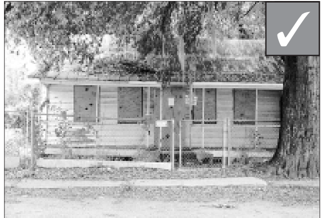
At times, it may be necessary to "mothball" a building in order to keep it safe until it can be improved.
