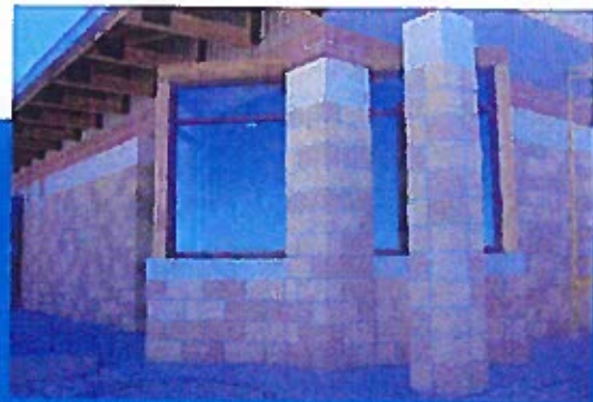
Electrical and Control Building at Lake Stillhouse Hollow Raw Water Intake Site
