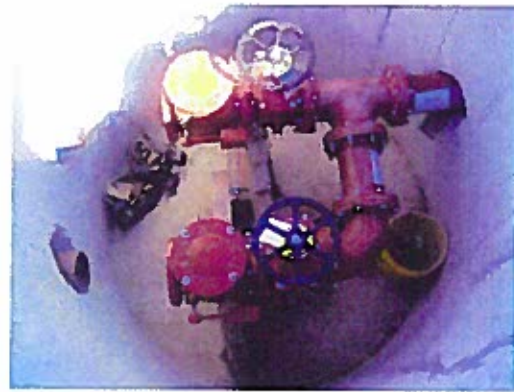
Wetwell and Piping for Supernatant Return Pump Station
