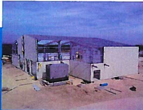
Treatment Plant Metal Building, Emergency Generator
