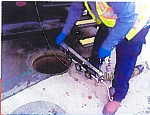
Wastewater Manhole will be Entry Point to Televising Existing Wastewater Line to Inspect for Possible Damage
