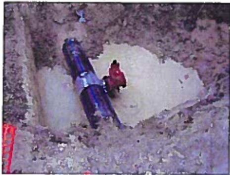
Tee and Gate Valve on Polyethelene Pipe
