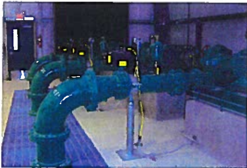
Membrane Filtration Pump Discharge Piping Turning into Floor Piping Chase
