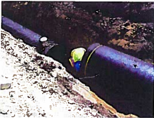
30" Ductile Iron Raw Water Line
