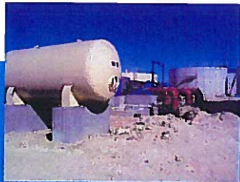
Welded Steel Hydropneumatic Pressure Tank on Concrete Foundation Adjacent to Pump Station Foundation. Tank and Pumps Provides Plant Water Service
