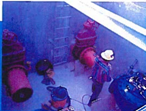
Piping and Valves in Surge Relief Valve Vault
