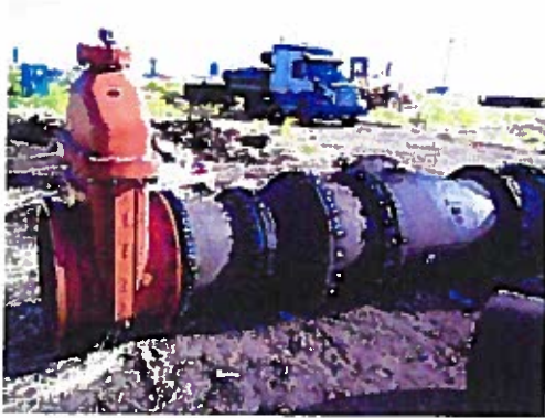
30" Ductile Iron Tee, 24" Gate Valve near East Amity Road at I.H. 35
