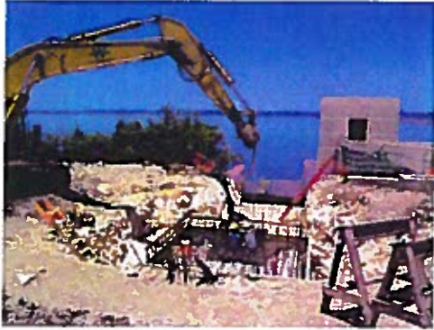
Surge Relief Valve Foundation, Existing BRA Raw Water Intake Structure and Lake Stillhouse Hollow in Background
