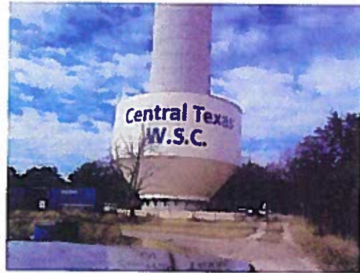
Tank Bowl Painted and Ready to Raise to Top of Concrete Structure
