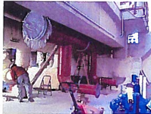
Piping for Two-New 4 MGD Raw Water Intake Pumps on Intake Structure, 30" Raw Water Piping Manifold
