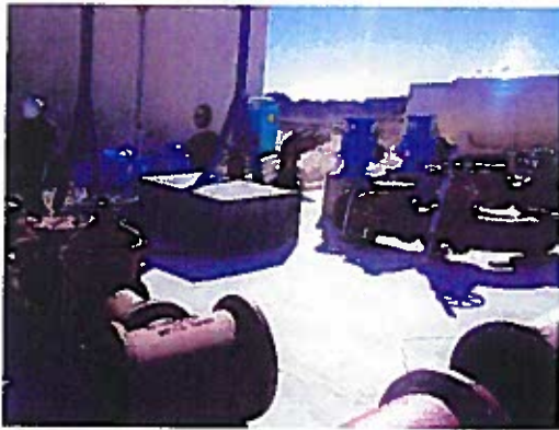
Concrete Pump Pads, Ductile Iron Piping Fittings in Pump Station Building
