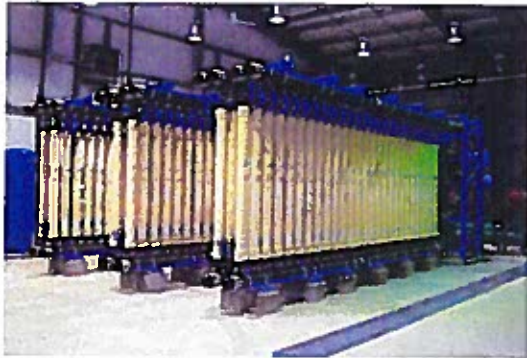
3 – 1.5 MGD PALL Membrane Racks
