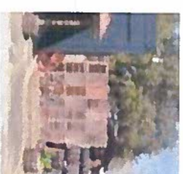
Removal of Shutter Wall and Lean to from right side of building
