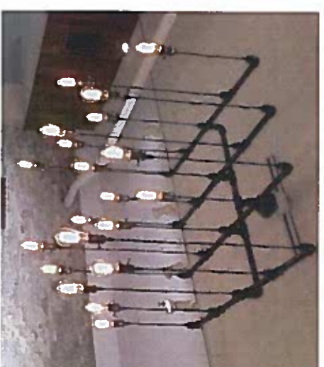
Industrial Lighting Fixtures
