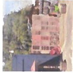
Removal of Shutter Wall and Lean to from right side of building
