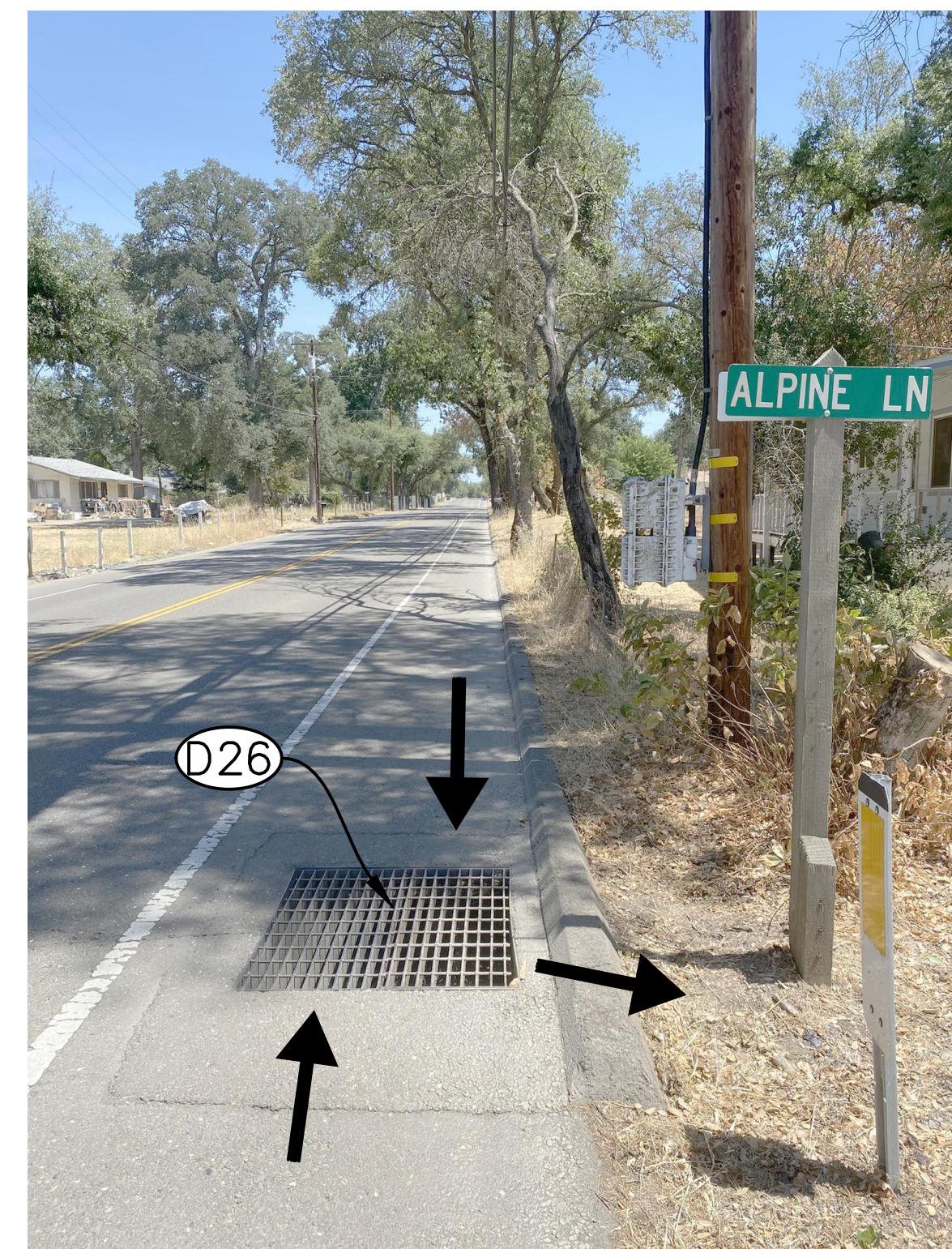
CATCH BASIN SOUTH OF KING ROAD (LOOKING EAST)
