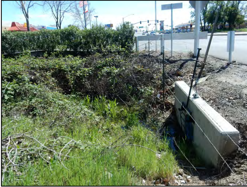
1. Looking at southwest corner of property at culvert carrying flows of WS-3 to the west under Sierra College Blvd. Photo date: 3-25-16
