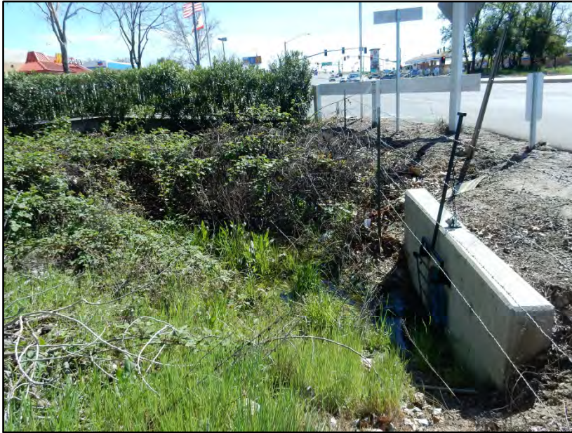
1. Looking at southwest corner of property at culvert carrying flows of WS-3 to the west under Sierra College Blvd. Photo date: 3-25-16
