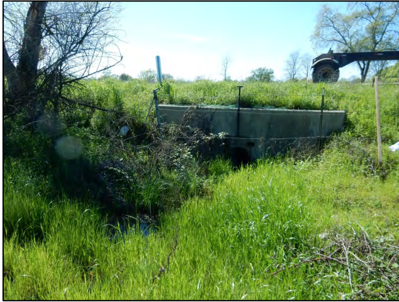
1. Culvert carrying flows to the west from WS-1 under Sierra College Boulevard. Photo date: 3-25-16
