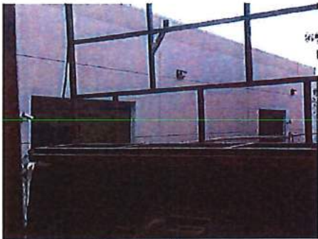
Bay Doors wide open
