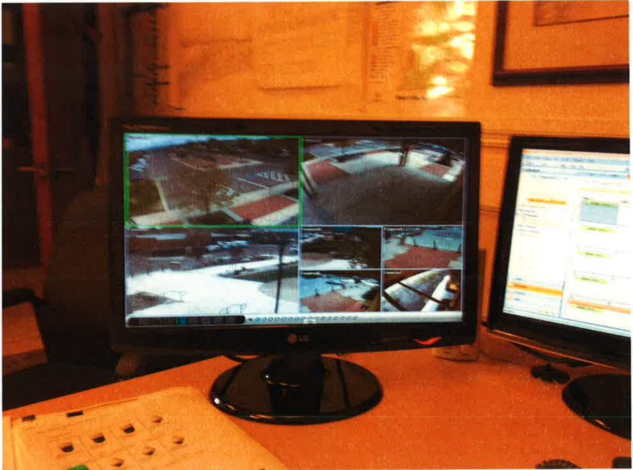
Figure 6 Security Camera Monitor
