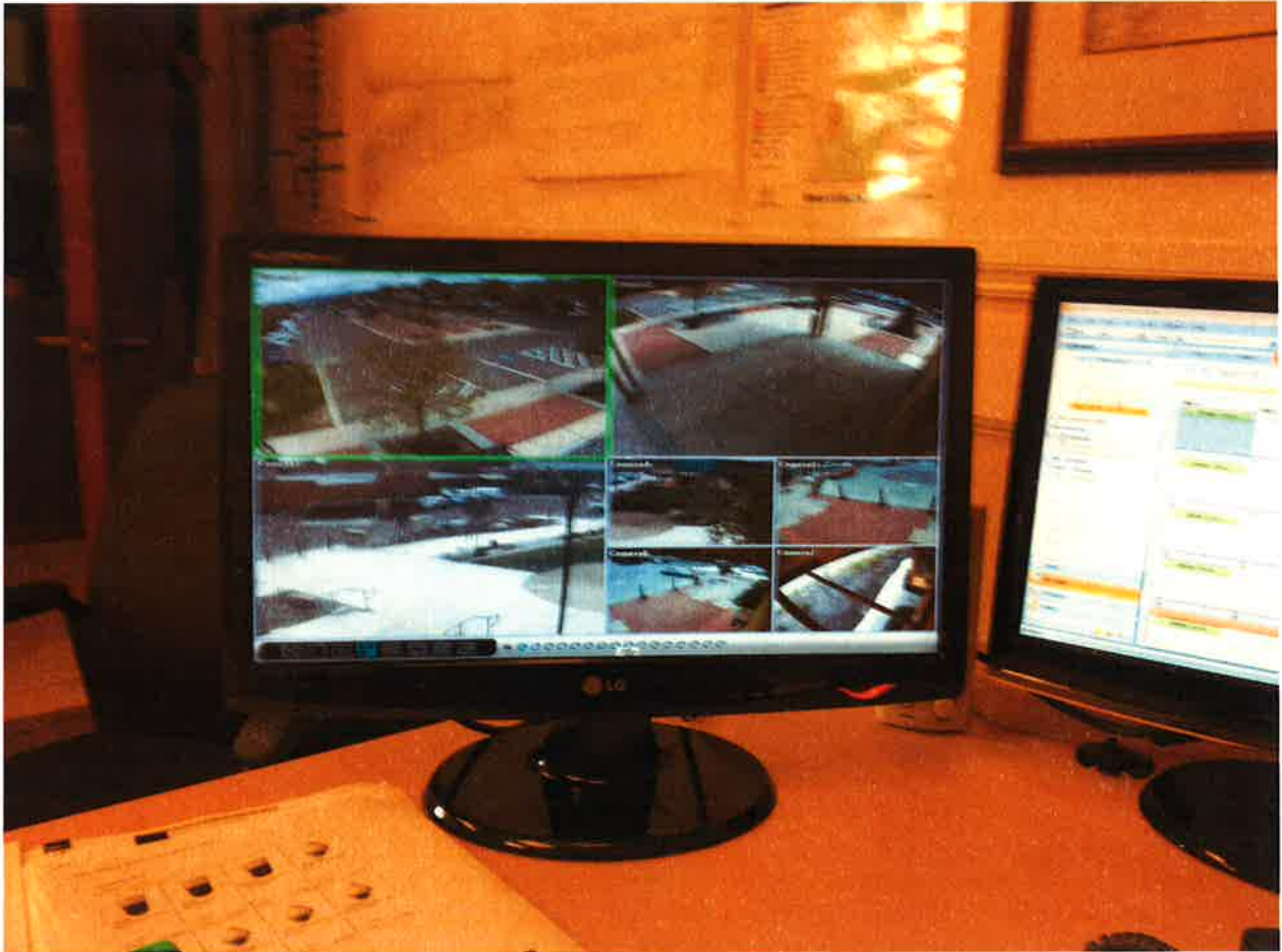
Figure 6 Security Camera Monitor
