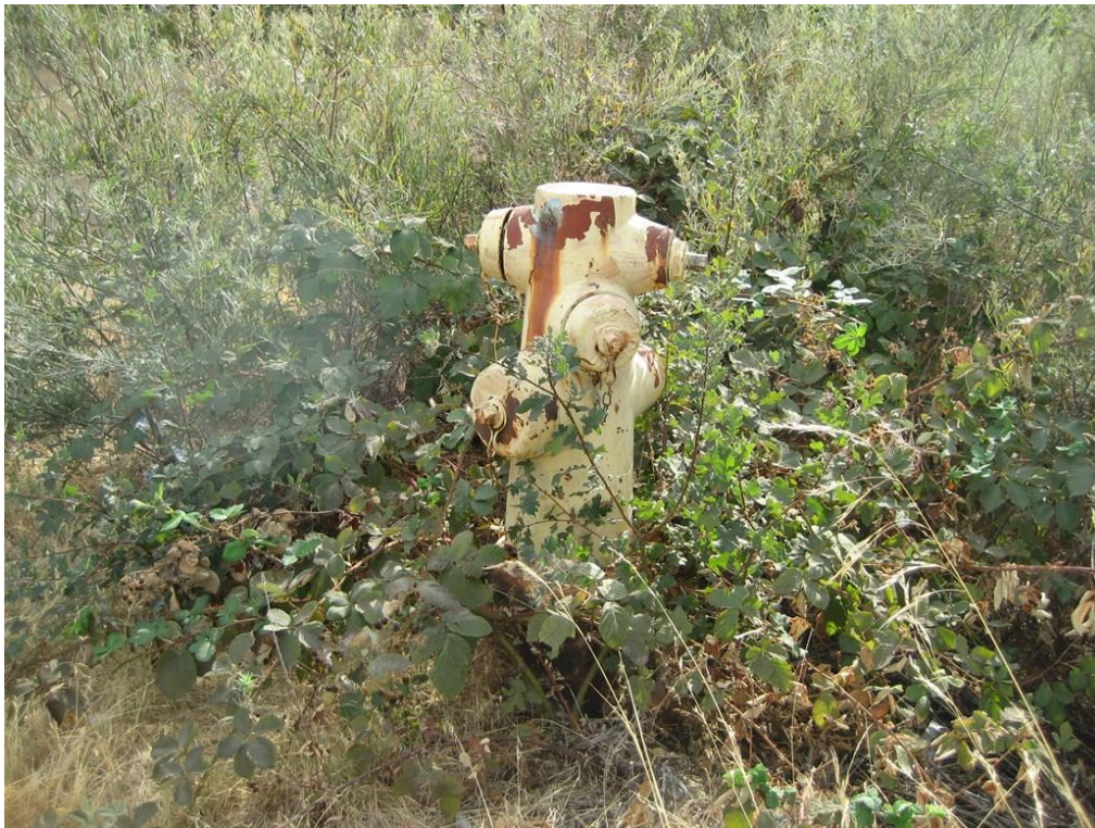
Photo 20: View of a fire hydrant located in the northeastern portion of the subject site adjacent to Sierra College Boulevard.
