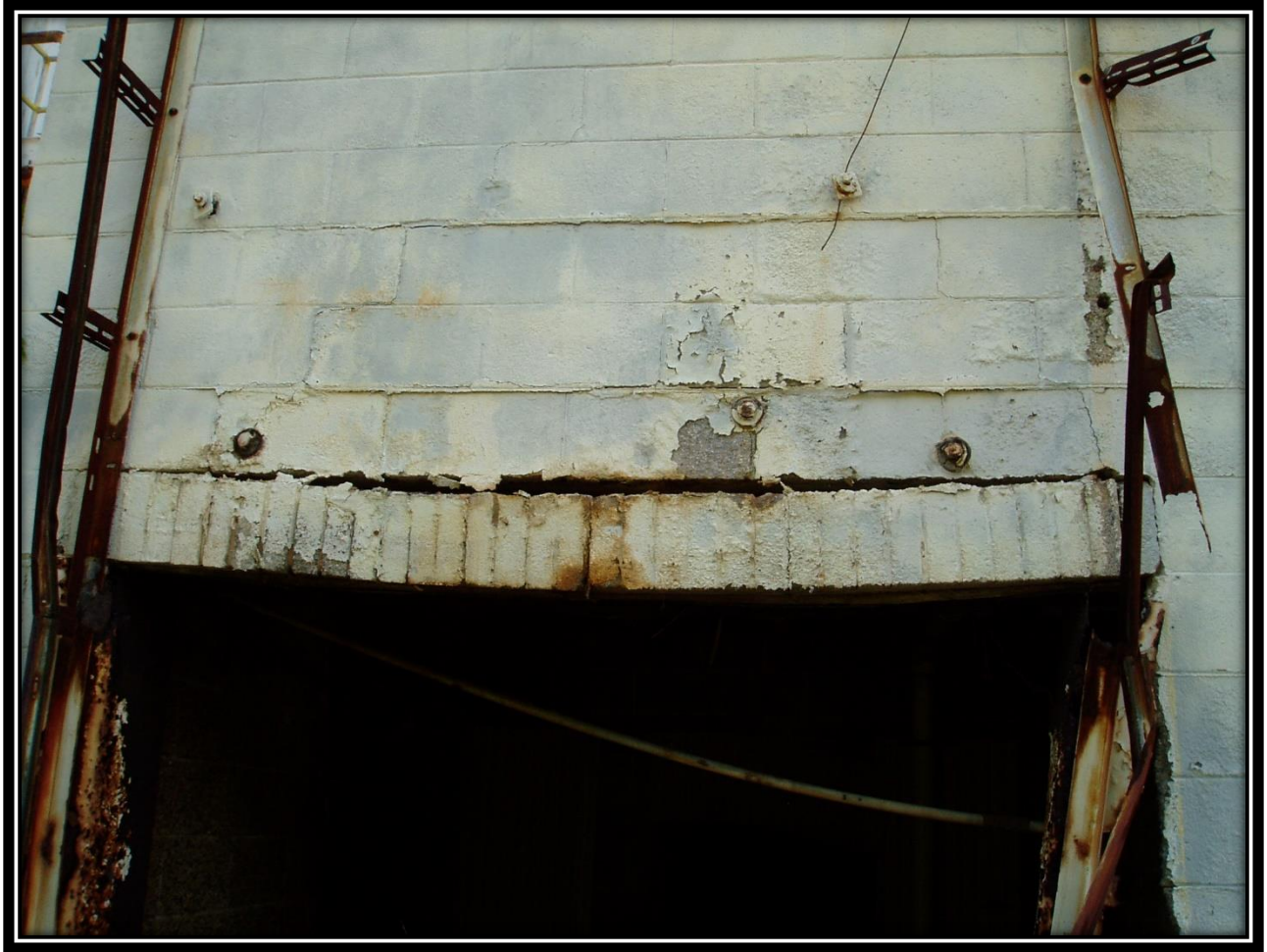
Bldg 5 – Lintel almost at failure. Avoid this back corner the building. Chemical attack on all building materials – steel, masonry and concrete.
