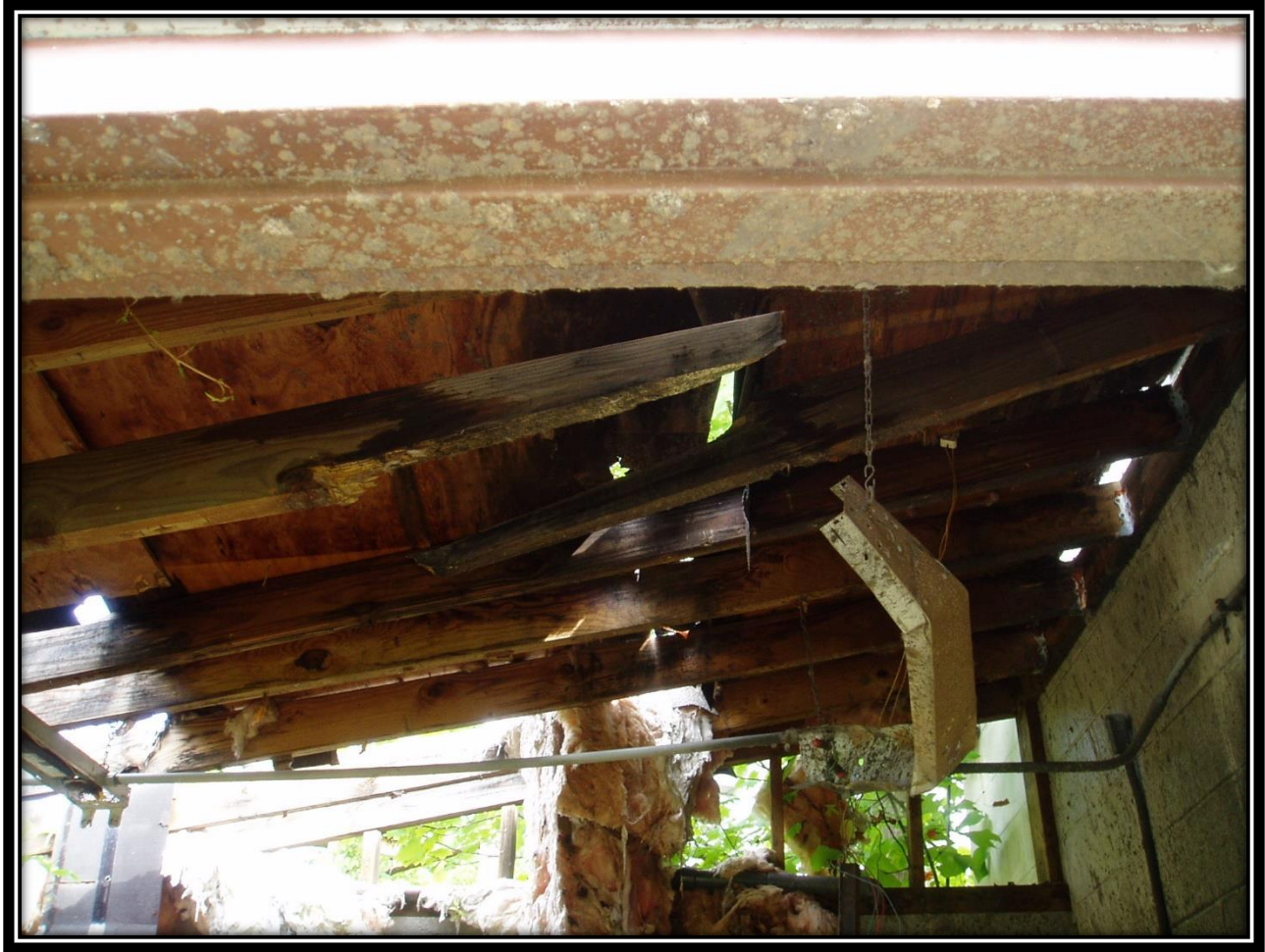
Bldg 21 – Wood framed lean-to on back of building should be avoided.
