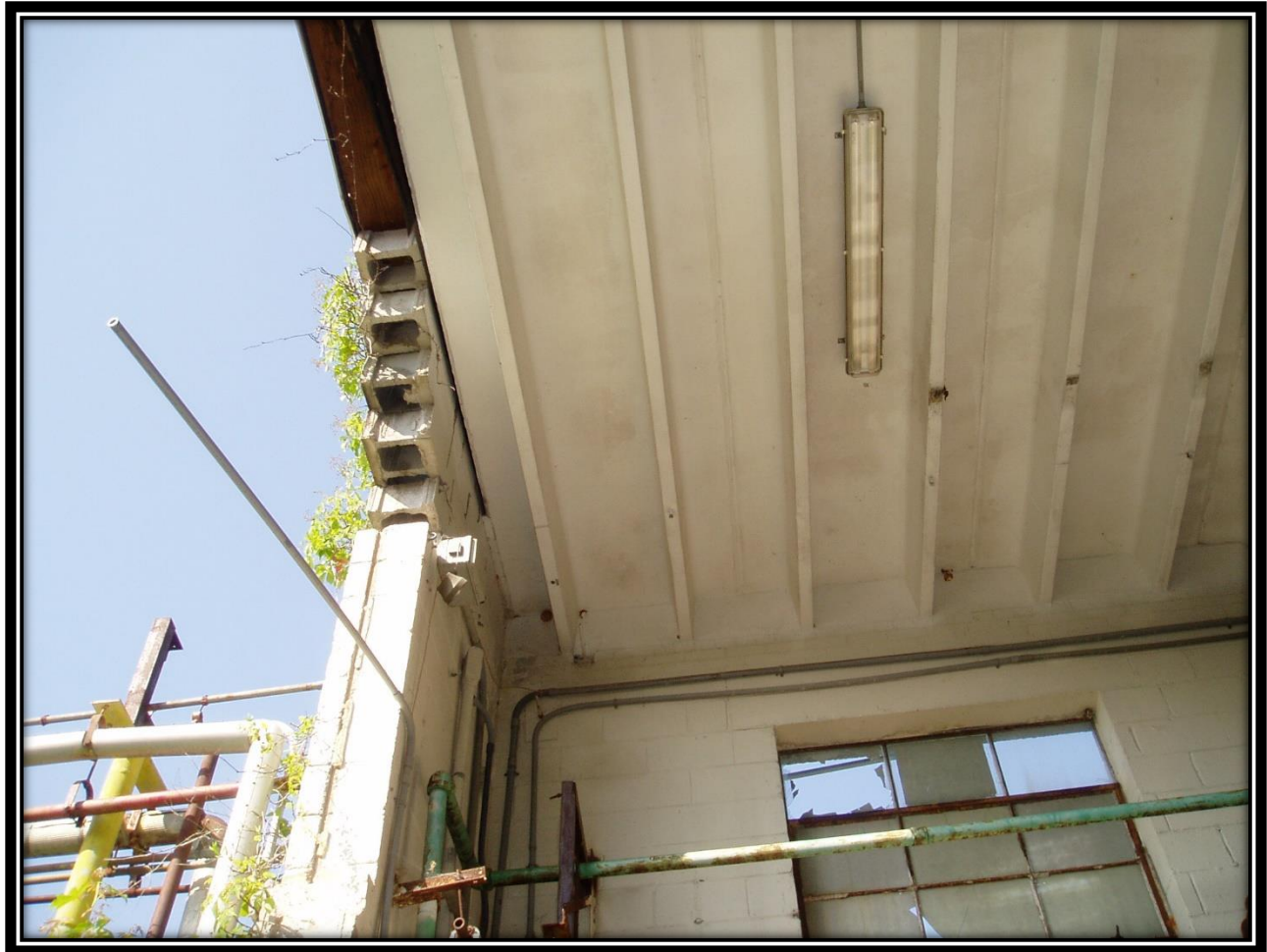
Bldg 10 – Hanging CMU pieces at entrance of building. Avoid this area in case they come loose and fall. This is a non-load bearing wall.
