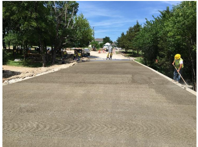
Looking north from the north side of the west Bridge as the new concrete is being placed and worked.
