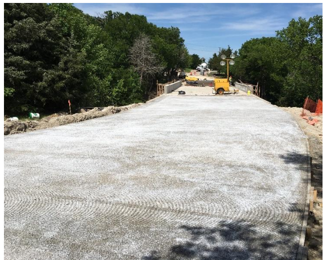
Looking north across the west Bridge after the south side pavement has been placed and has started to cure.
