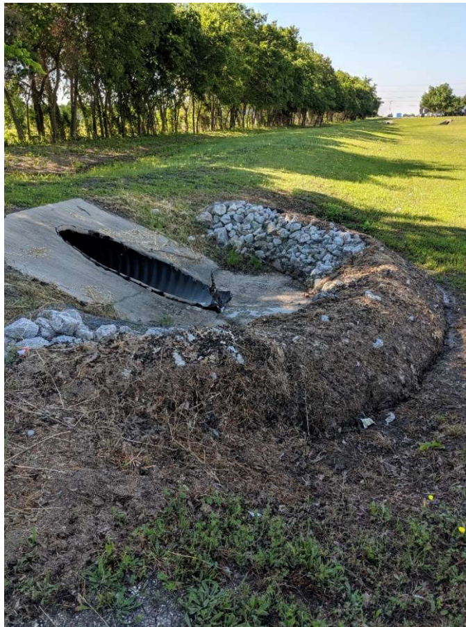
Image 2: Lovejoy High School Pond Outfall
