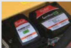
Diesel fired Beckett Burner
