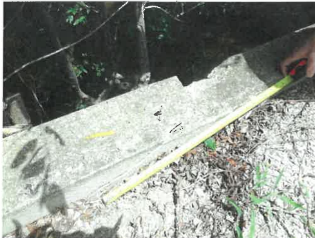
Crack and 8" x 5" x 2.5" spall at headwall 2, top, midspan
