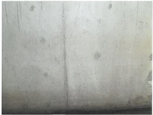
0.025" crack full height and depth through wall at 15'
