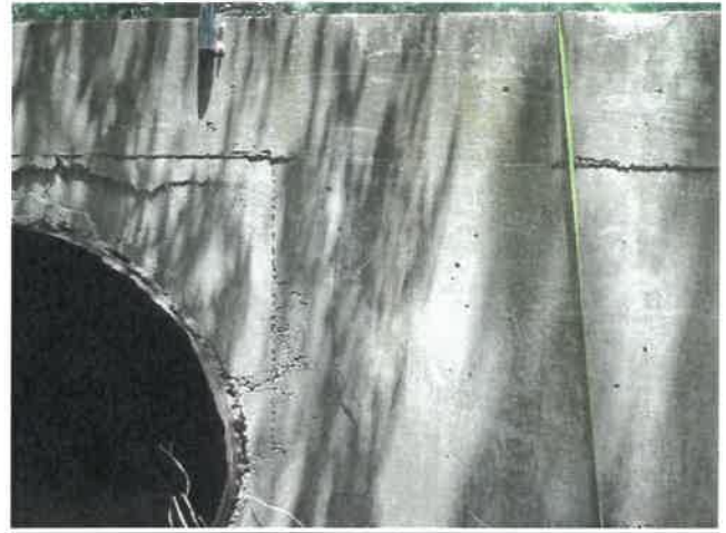
0.025" crack midspan headwall 1, full depth. crack continues approx. 7.5' down headwall
