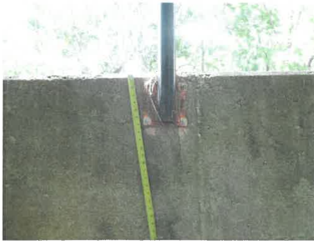
3" x .05" crack at first railing support connection to headwall 2
