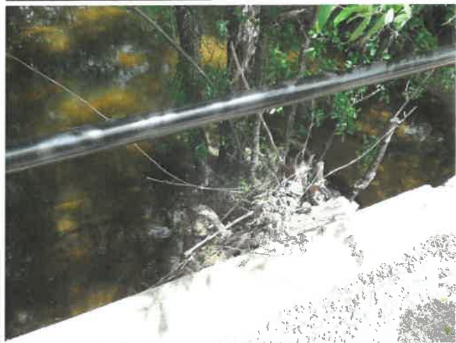
Evidence of flooding
