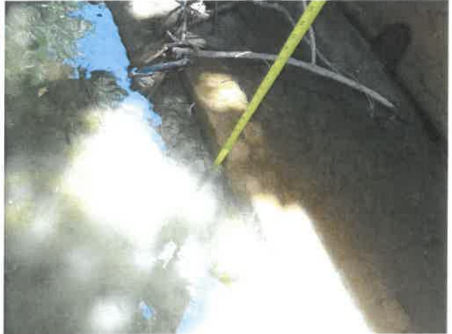
5" scour at bottom slab toe, northeast corner
