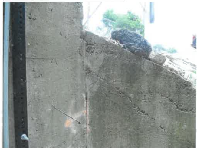
19" x 1/8" crack at wingwall 1
