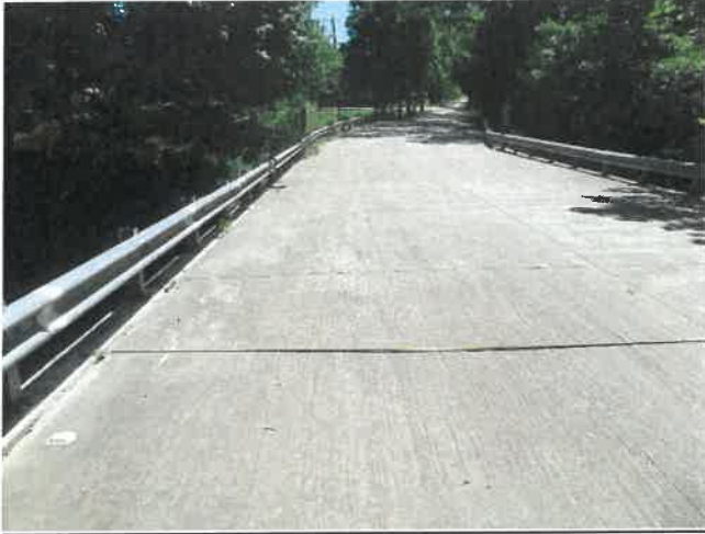
Lateral crack full width of roadway
