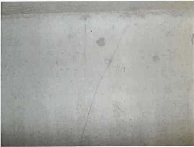
0.020" full diagonal crack center of bridge
