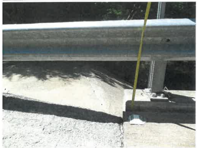
2-1/2" settlement of approach slab 2
