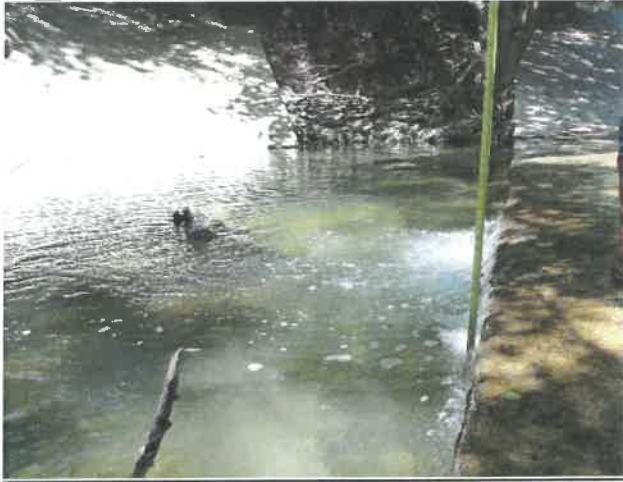
Exposed bottom slab toe with 18" scour and undermining at south outfall
