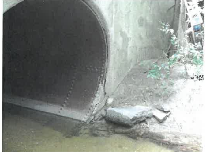
Spall at headwall 2, culvert 1 (Likely resulting from construction)
