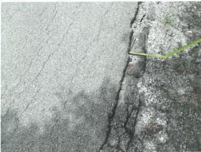
Asphalt Pavement edge failure in all four corners (Typ.)
