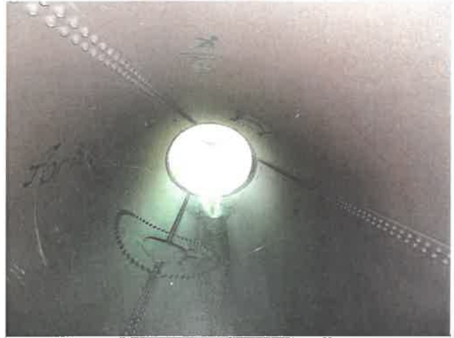
Moderate corrosion and sediment build up along bottom
