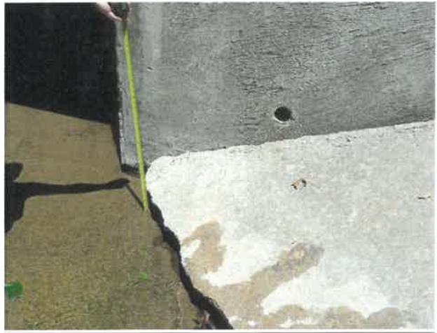
Toe exposed; chipping and undermining of riprap
