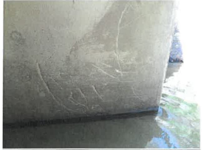
Scarring and gouging from debris at northwest corner (Typ.)
