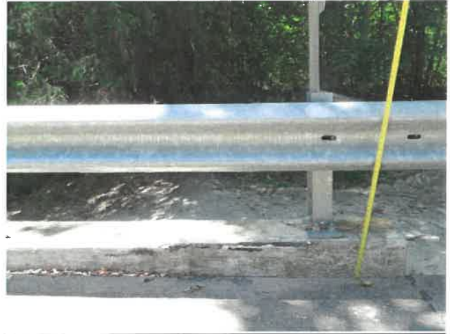
6" settlement of approach slab in southwest corner
