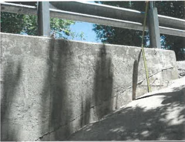
Concrete riprap settled 9"
