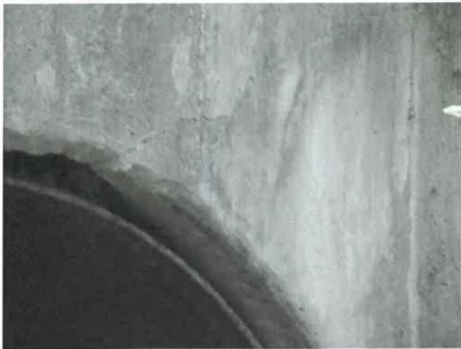
5' Horizontal crack near culvert 1
