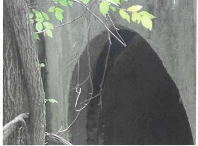
Scour/erosion at outlet headwall above pipe. Loss of backfill
