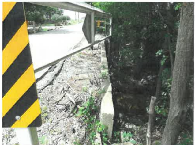
Headwall 2 out of plumb
