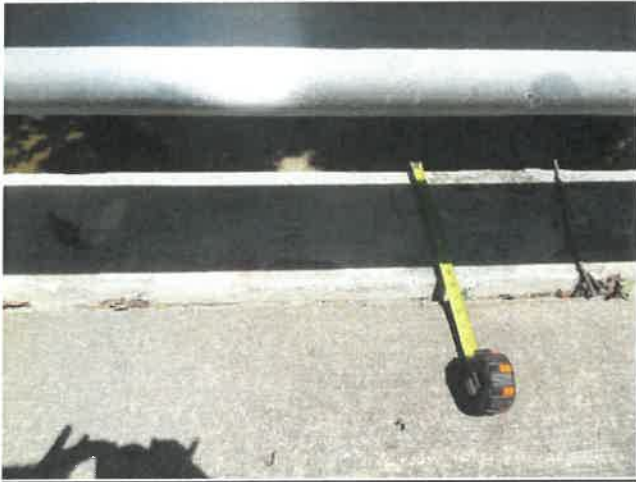
Full width hairline crack at the beginning of span 3
