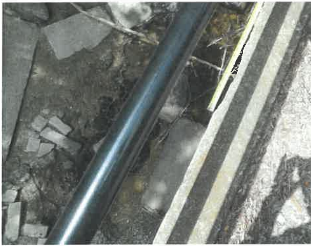
10" x 4" x 1" Spall midspan
