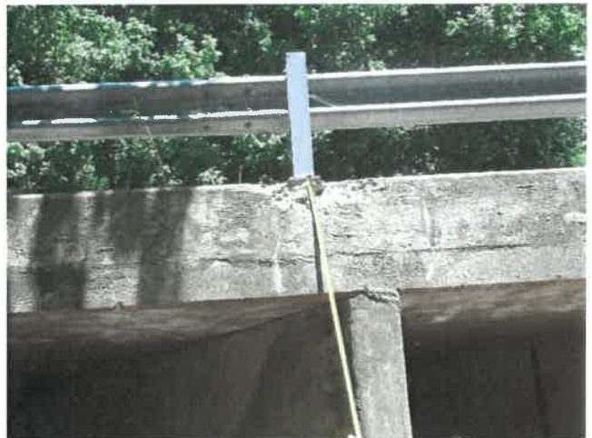
15" X 3" spall at both posts on span 2 (Typ.)
