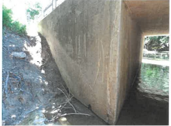
No slope protection; scoring and gouging from debris (Typ.)
