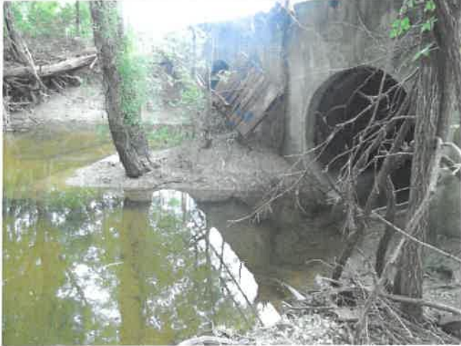
Approximately 1 ft scour at outfall and exposed encased utility
