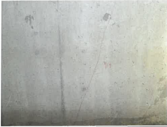
0.025" crack full height and depth through wall at 12'
