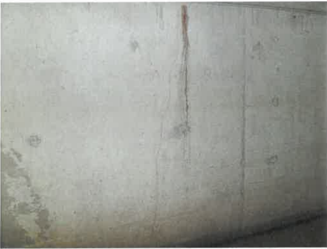
0.010" crack full height at 10' with efflorescence
