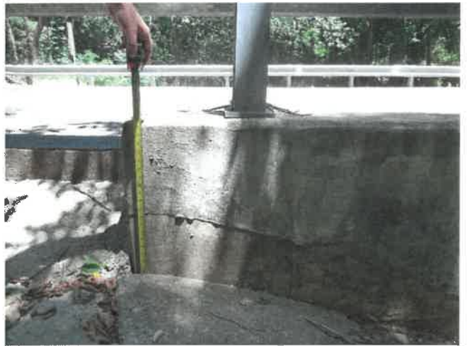
Slope protection appears to have settled 8" at southwest corner
