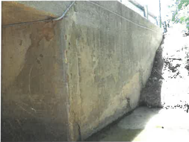
No slope protection; 1/8" full height crack and spall; moderate bank erosion
