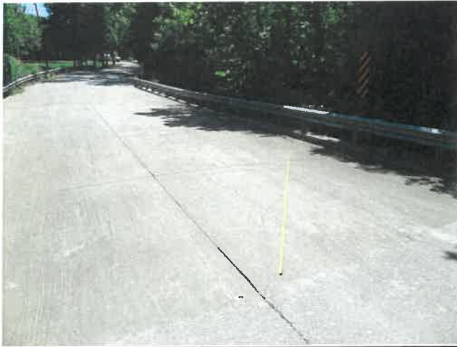
Diagonal crack at southwest portion of approach
