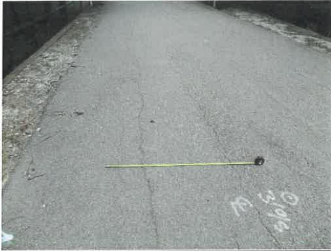
Left lane with Marginal longitudinal cracking (Typ.).
