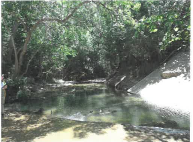
Moderate bank erosion looking downstream
