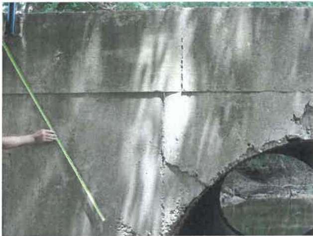
Spall and 6' x .030" crack north of culvert 2, headwall 1
