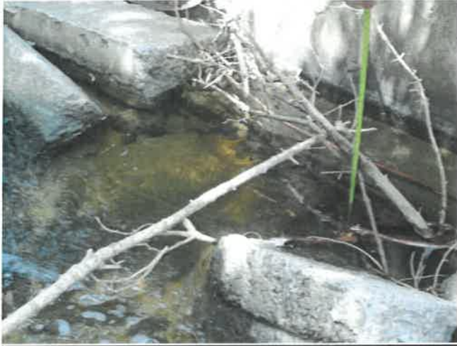
Undermining of headwall 1 at midspan
