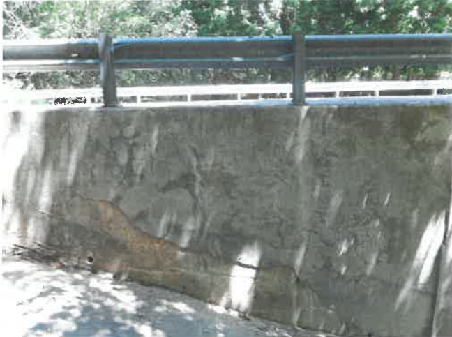
75% delaminated on southwest face abutment 1
