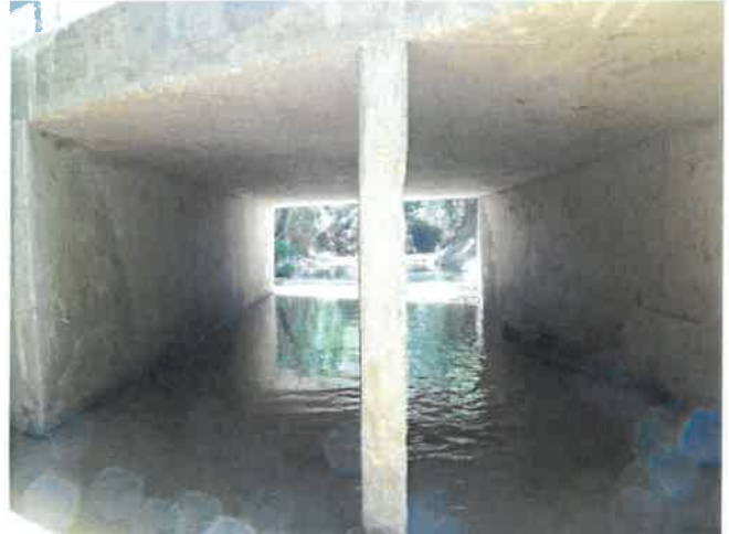
20" x 7" x 1" spall (varies) (likely from debris impact)
