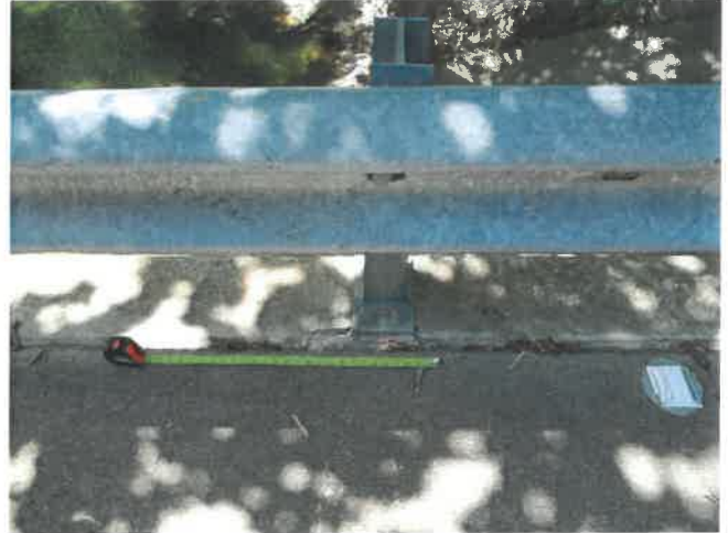
2" x 13" x 1" spall at second railing post of span 1
