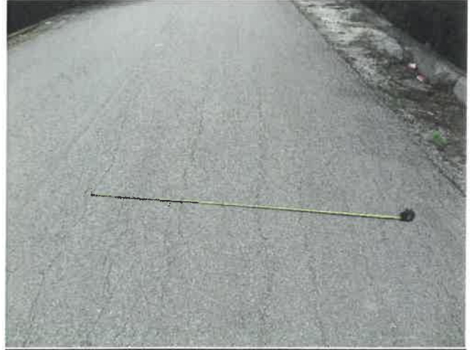
Right Lane substantial longitudinal cracking.
