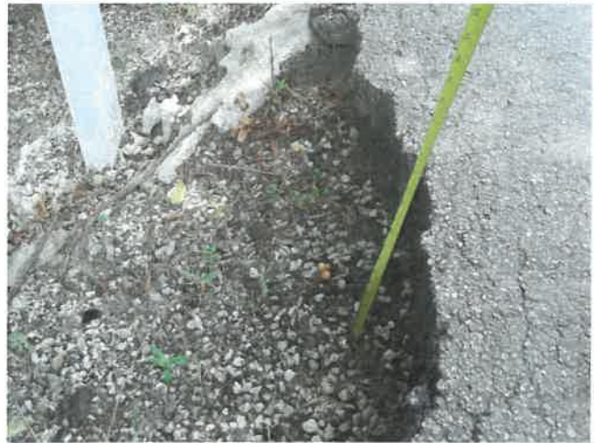
Substantial pavement failure (12")
