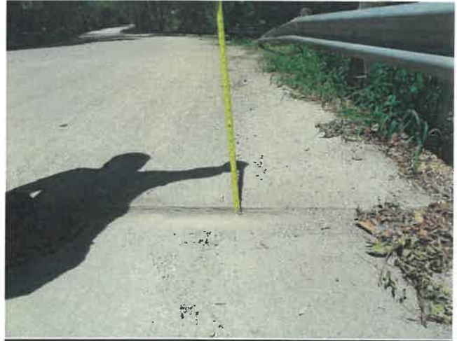
Approach slab settled 1" at roadway
