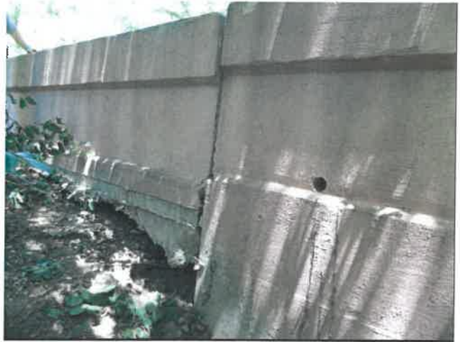
Scour and undermining both sides
