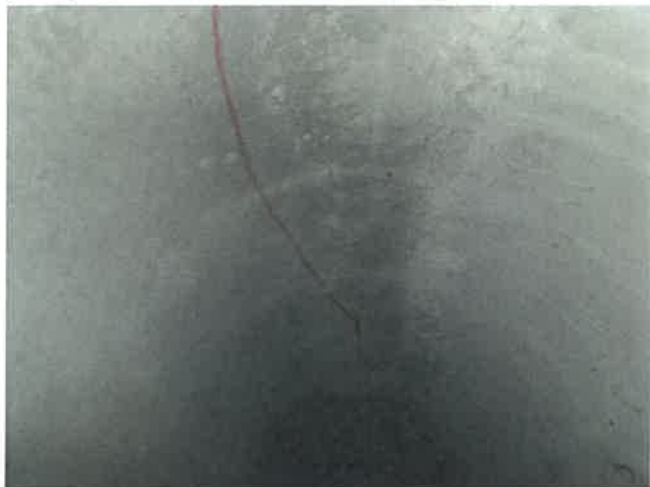
Longitudinal crack bottom of deck between beams 8 and 9
