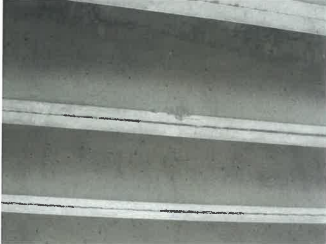
6" X 3" X 1" Spall at beam 10 7' from bent 2
