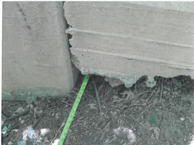
At least 13' of undermining under approach slab of northeast corner
