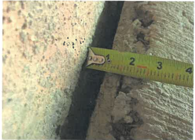
Concrete riprap settling away from abutment 7/8" (recommend Seal)
