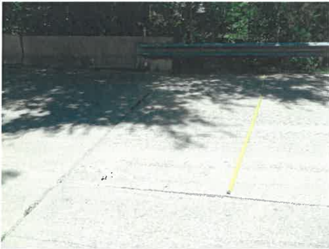
3'-6' Transverse cracking caused by approach slab settling on roadway
