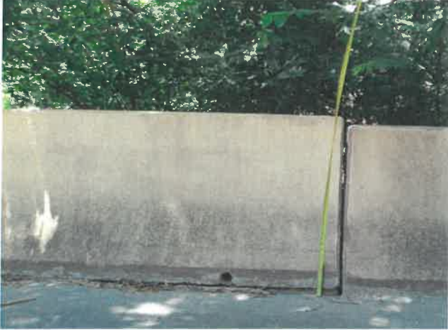
Approach slab settled 1-1/2" at northwest corner of approach roadway
