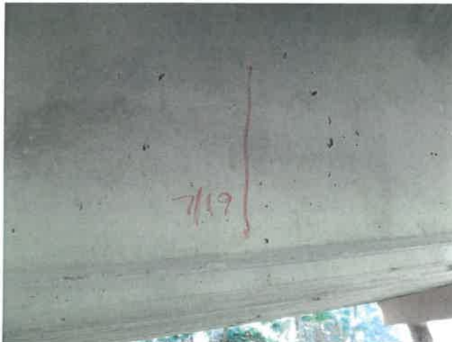
Hairline vertical cracks on beams 3, 6, 8, 9, 12 of span 1 (typ.)
