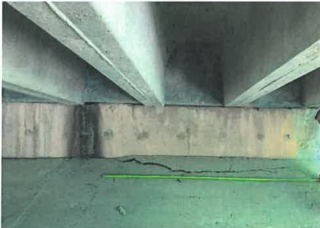
7' x 1" crack along concrete riprap & starting at abutment
