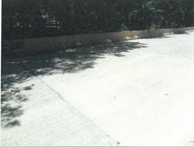
Southwest corner approach slab settled 1"
