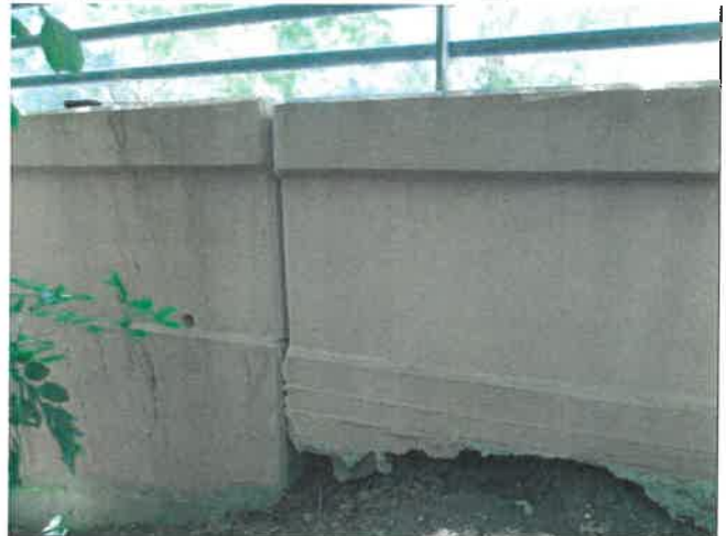
Northeast corner approach undermined (Typical both approach slabs, both sides)
