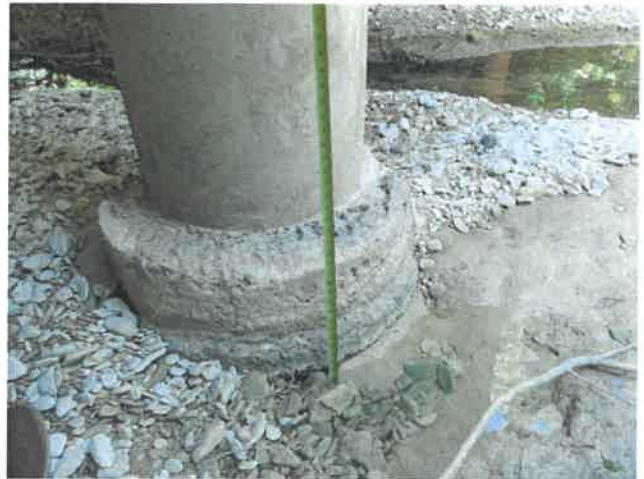
Exposed drill shaft from scour 13" (Typ.)
