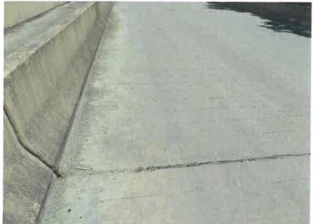
Shrinkage cracking along deck (Typ.)
