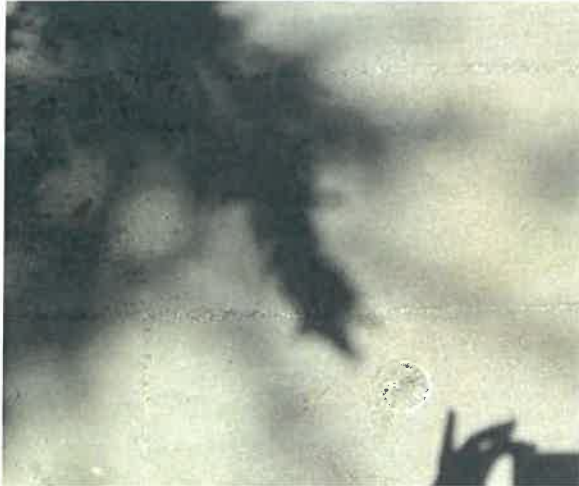
Scupper clogged mid span of span 1
