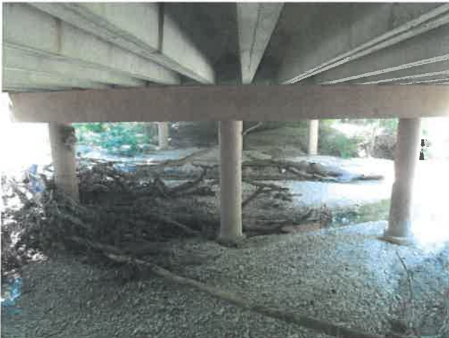
Evidence of flooding
