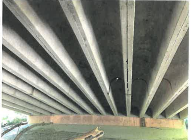
Longitudinal cracking under deck span 3 (Typ.)
