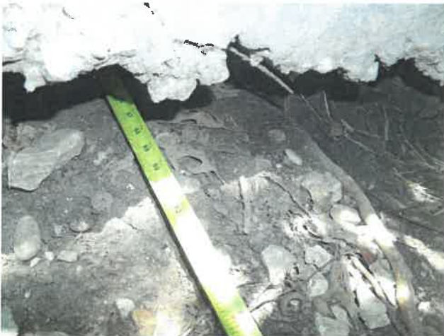
At least 8' of undermining at the approach slab
