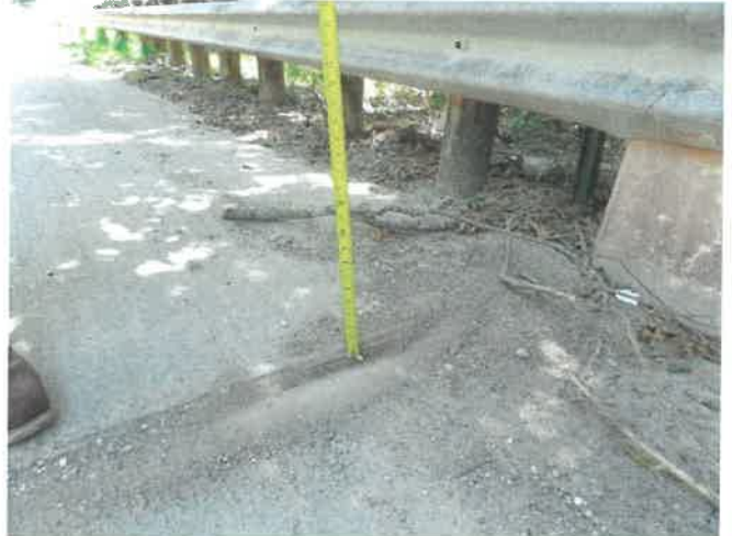
Southeast approach slab settled 1/2"
