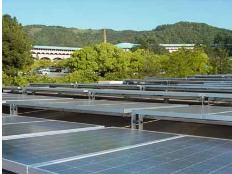
Demonstrating sustainable practices such as installation of solar panels on County facilities
