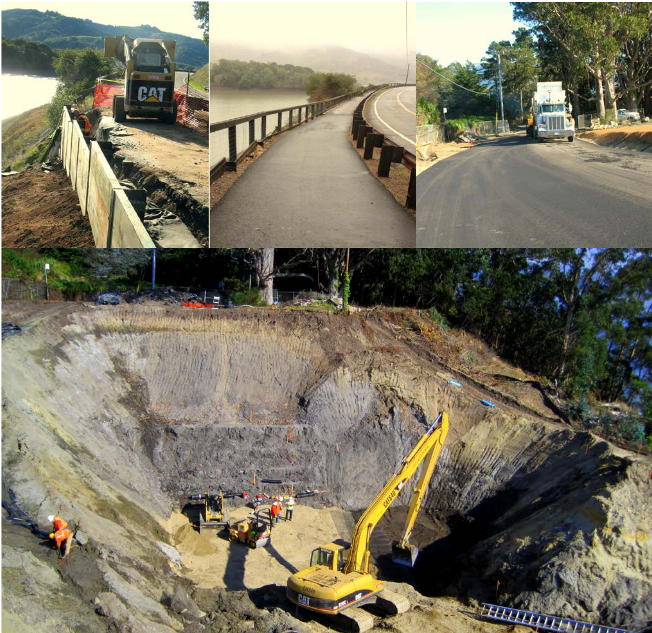
Slide Repair Projects at Stafford Lake and another on Terrace Ave/Overlook Drive in Bolinas.
