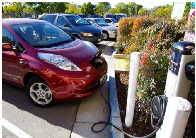
Electric Vehicle Charging Station at Civic Center
