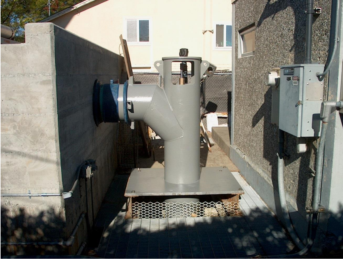
New Pump and Concrete Afterbay at Pump Station No. 2 in Santa Venetia
