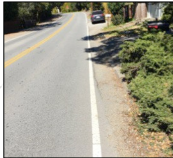
e) Unrideable gutter; encroaching landscape
