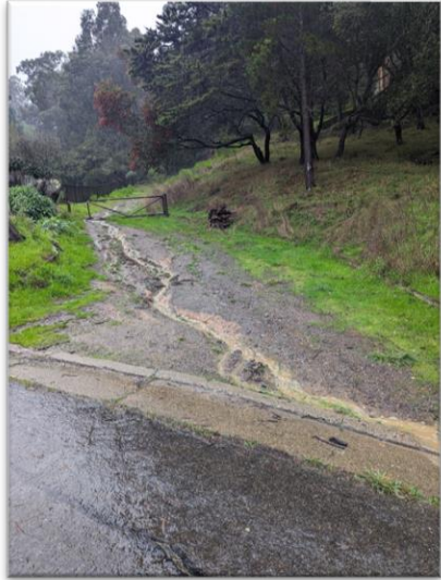
Fire road erosion
