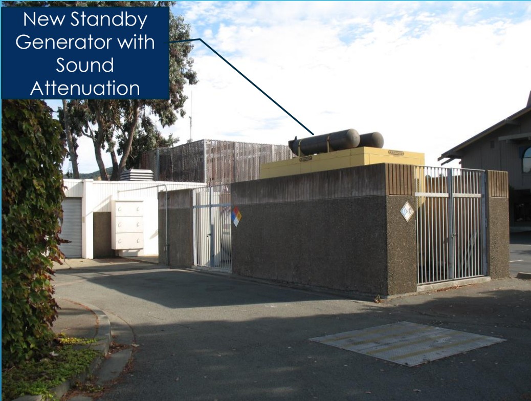
North Francisco Blvd Pump Station
