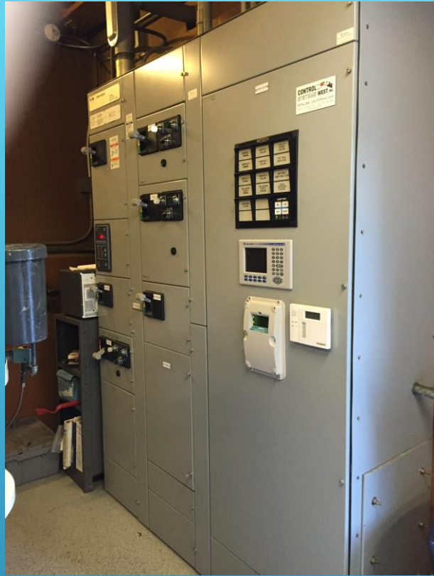
Motor Control Center
