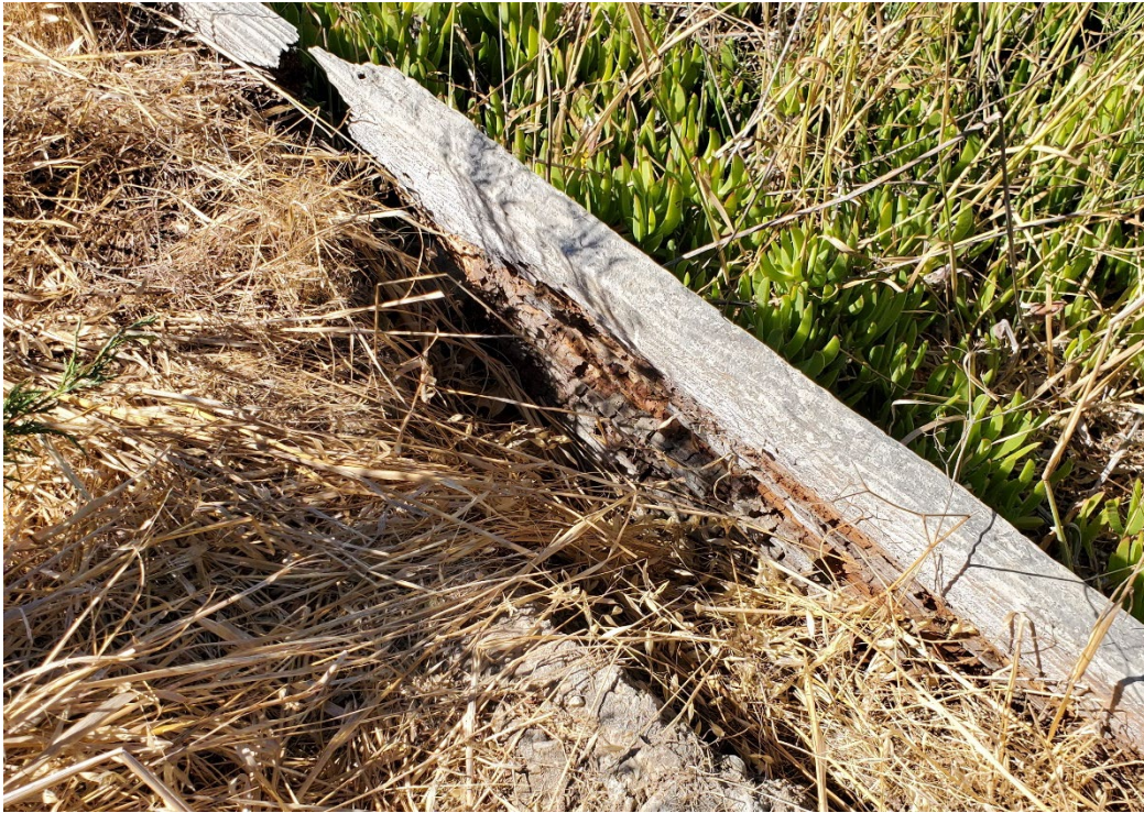
Figure 2-5: Loss of Soil Within TRB and Timber Deterioration
