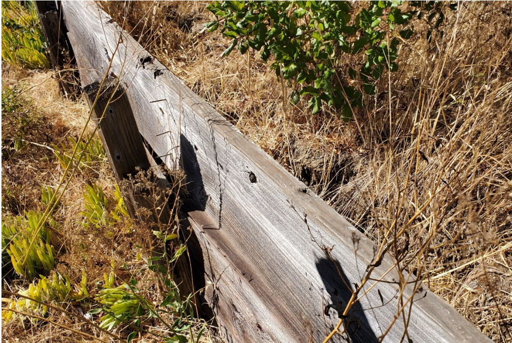
Figure 2-2: Deteriorated Timber Reinforced Berm
