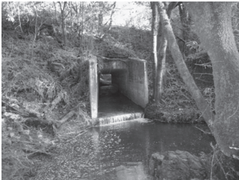
Traditional box culvert with concrete bottom
