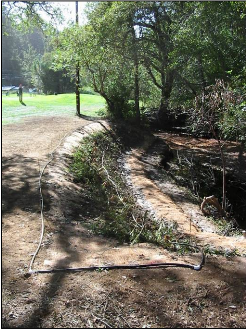
Biotechnical bank stabilization using gently-sloped banks and brush mattress. Note narrow bench created next to active channel. Photo by Prunuske Chatham, Inc.
